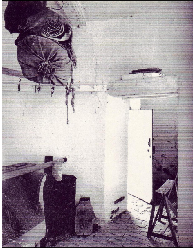
Looking into what is now the shower room, but was formerly the only entrance to the ground floor room.
