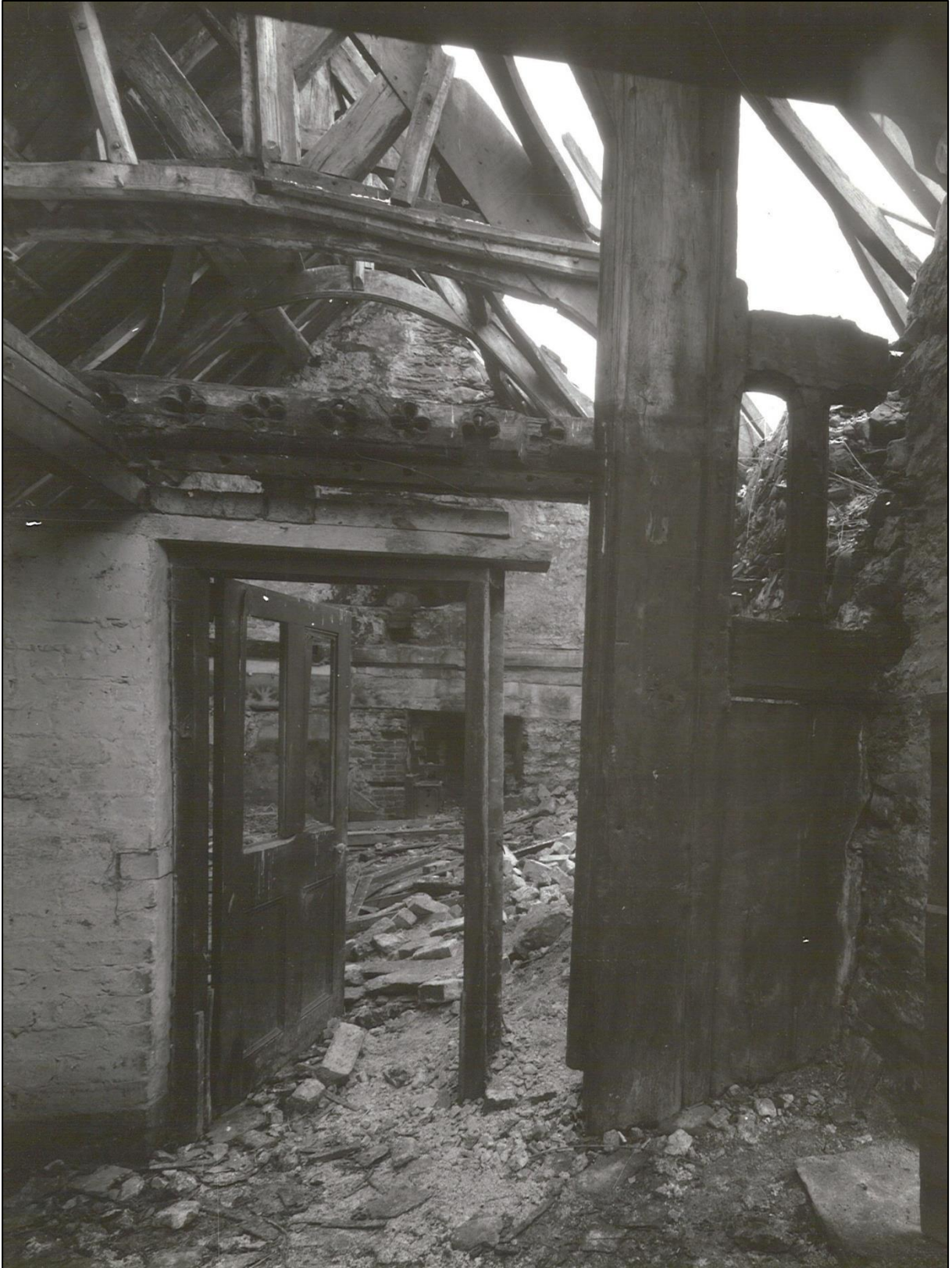
Interior in 1970, showing the spere truss and the beam linking the two aisle posts (RCAHMW).
