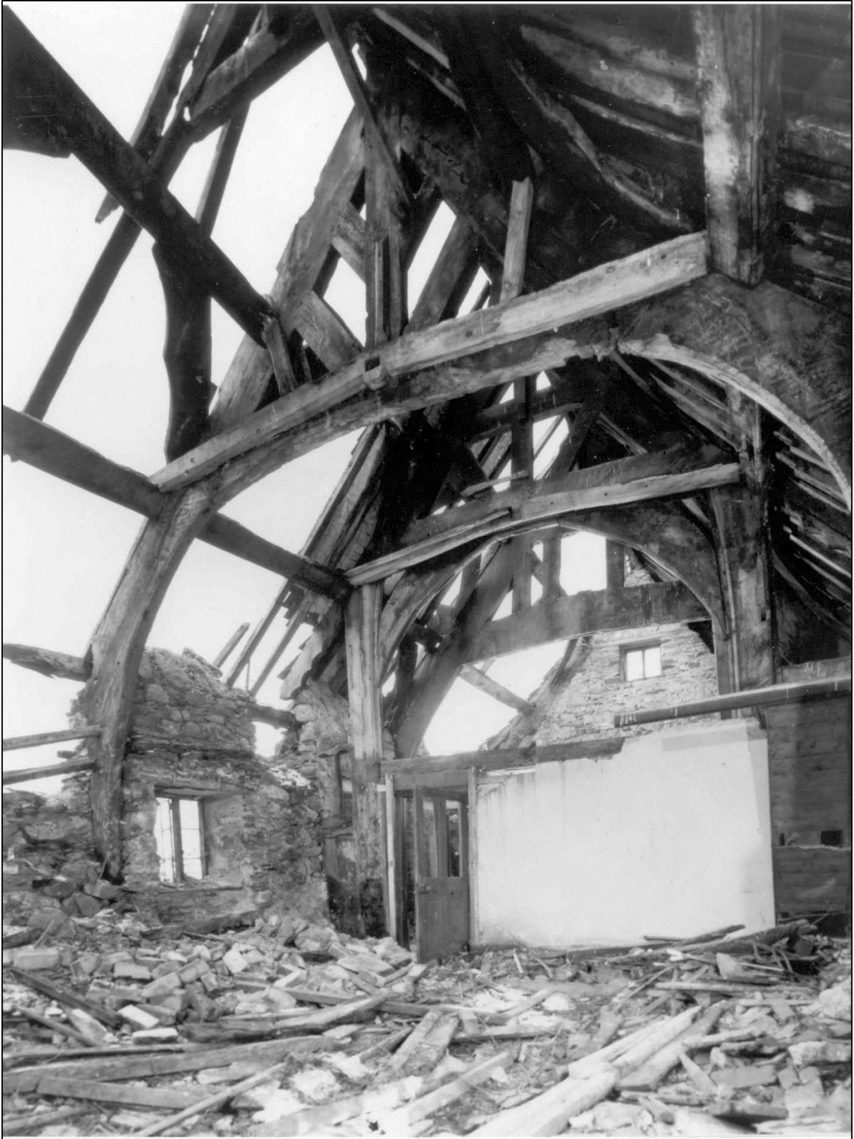
Interior in 1970, showing the extent of disrepair (RCAHMW).
