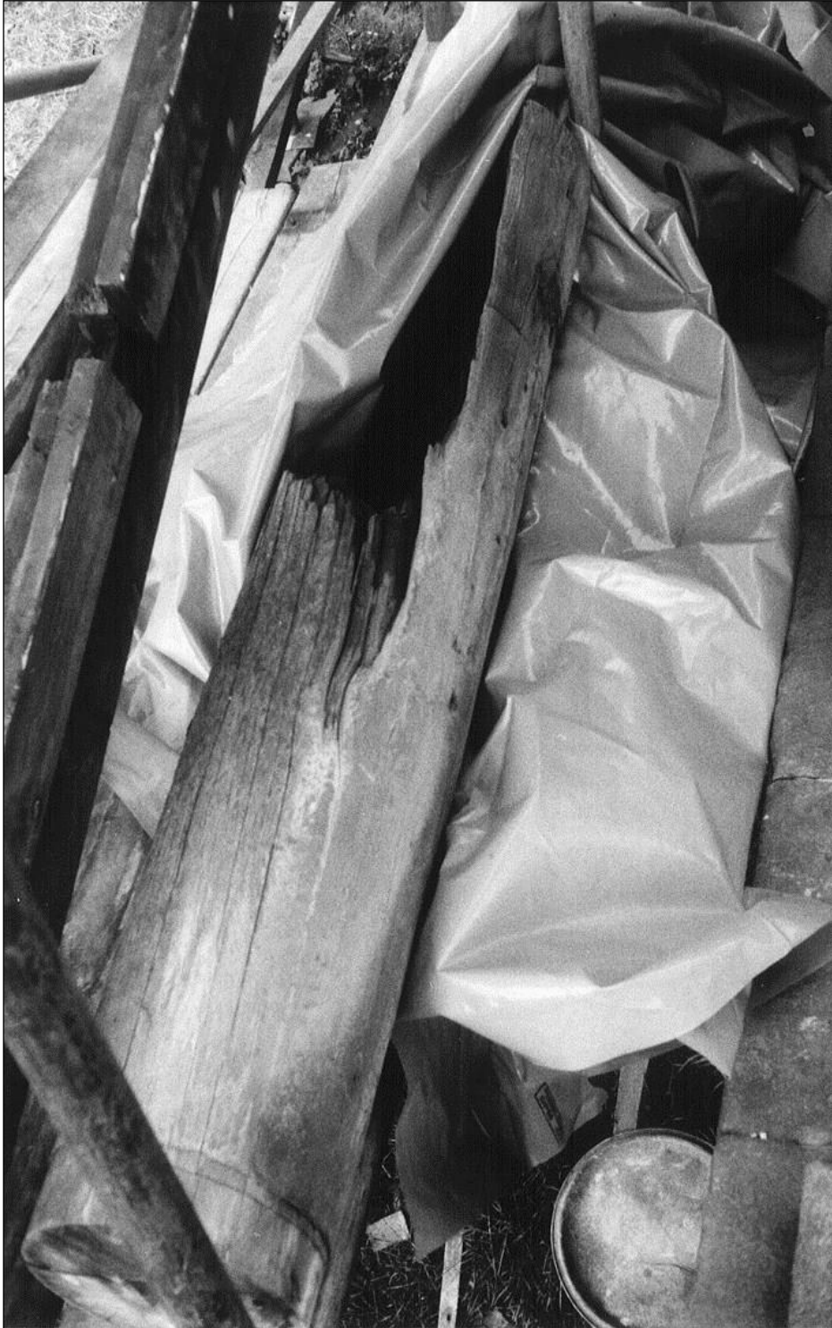
This column was too rotten to save, but helped to prevent the polythene from blowing away.
