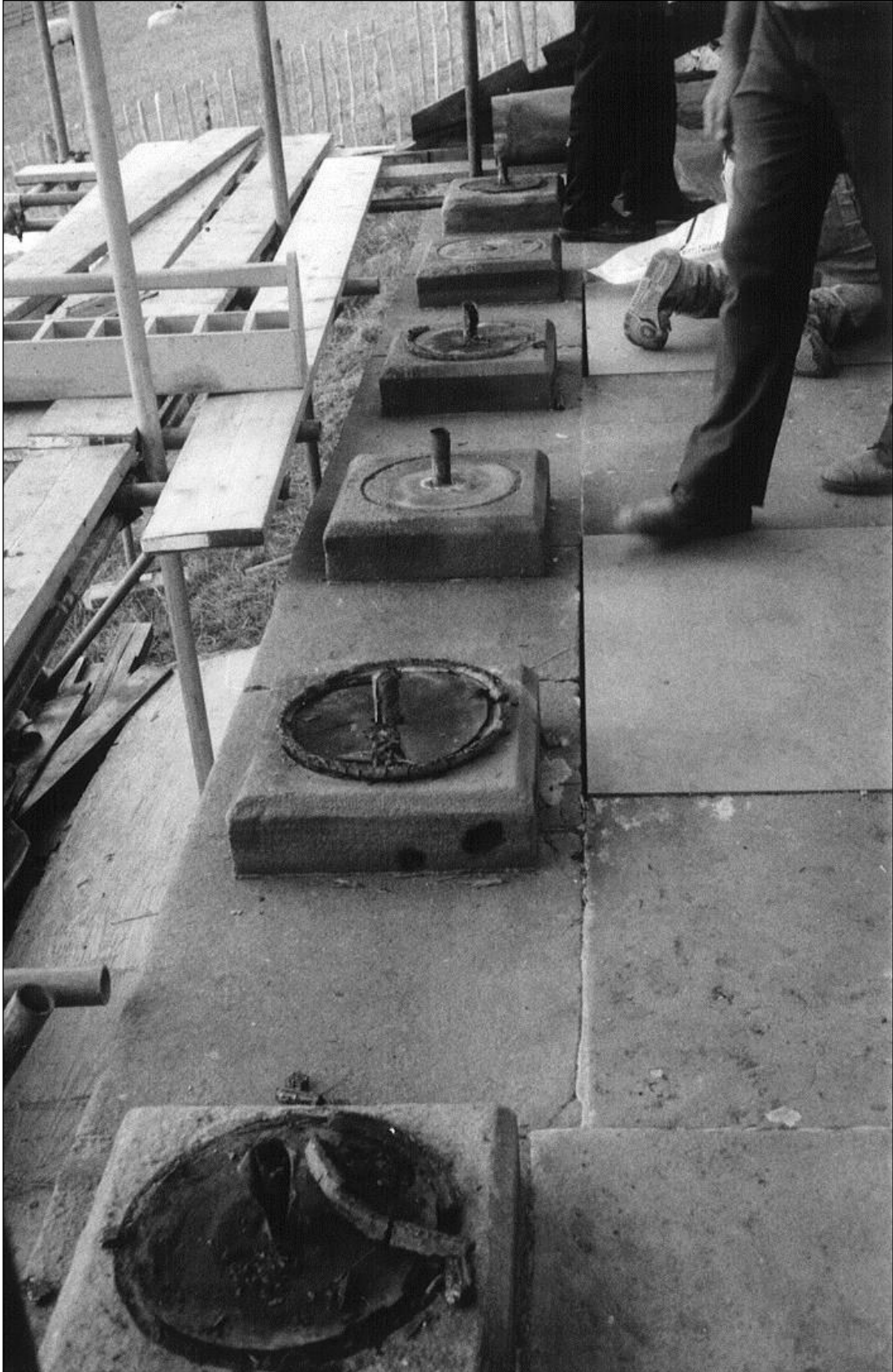
The bases of the columns after the portico was dismantled, and taken away for repair.
