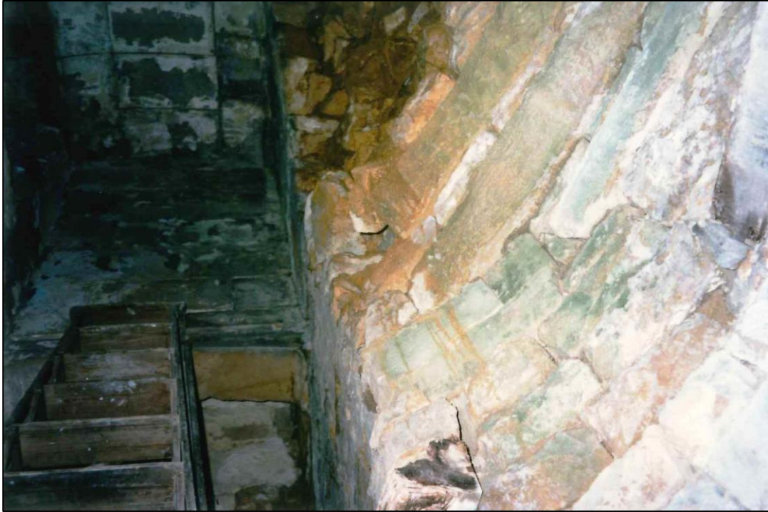
The collapsed staircase caused by water ingress.
