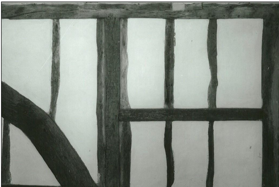
The south wall of the single bedroom was originally an outside wall. The framing shows the position of the earlier window. (RCHME)
