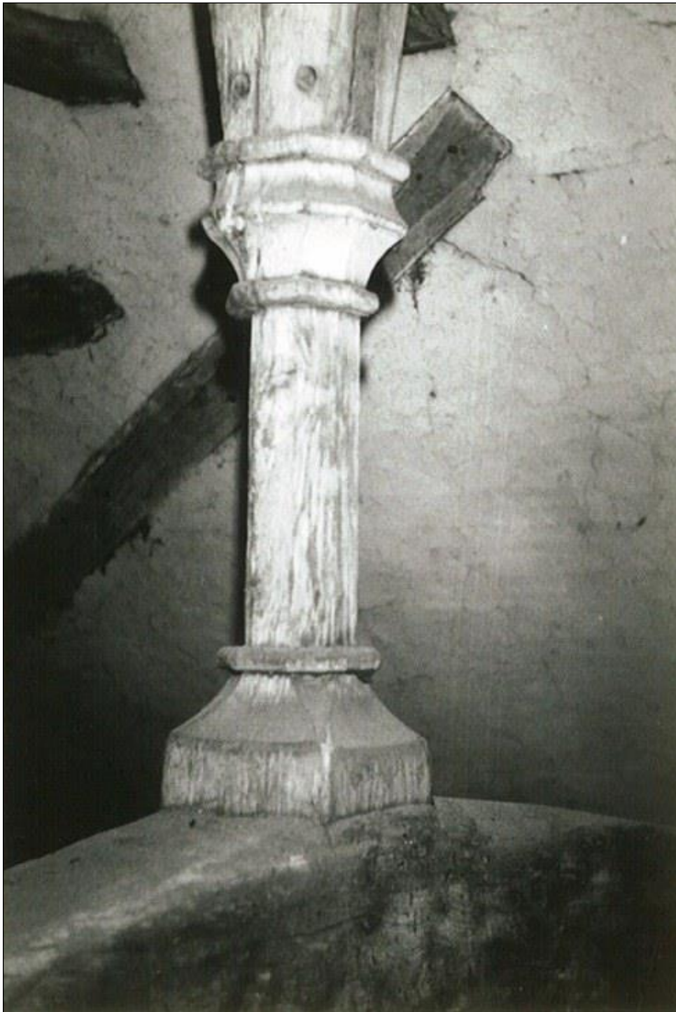
Crown post in the high end chamber prior to restoration. The crown post at that time was completely concealed from view by a ceiling inserted below the tie beam, so it was an exciting discovery.
