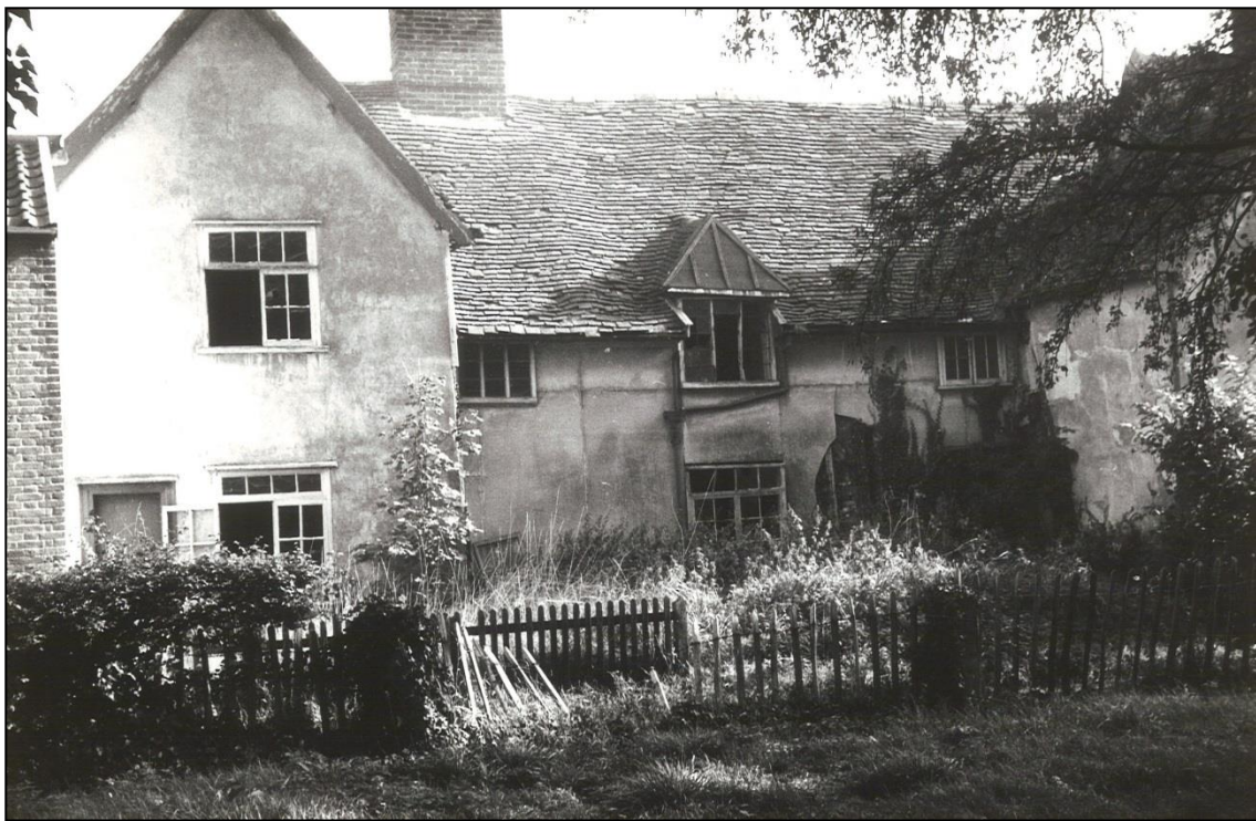
New Inn in 1971, by now known as Knoll Cottages. Its medieval character is hardly apparent behind later render and inserted window frames.
