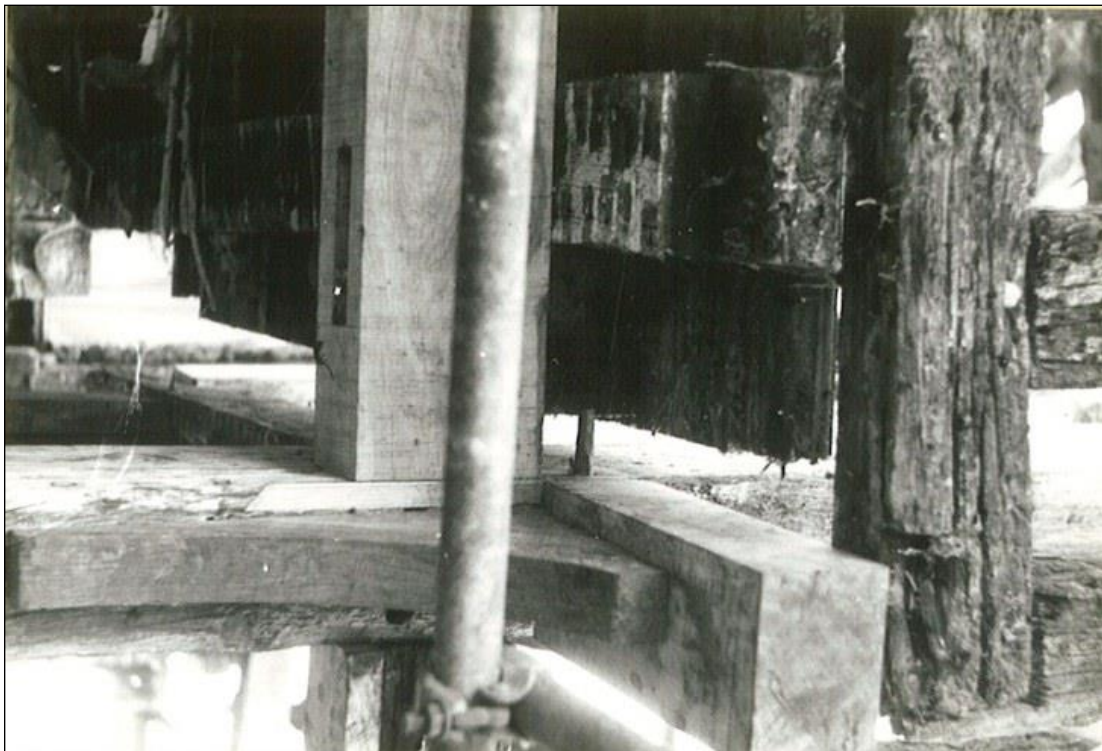
New timbers and bracket inserted beneath the jetty at the high end.
