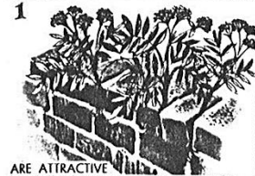
1 ARE ATTRACTIVE BUT VERY DESTRUCTIVE TO MASONRY
