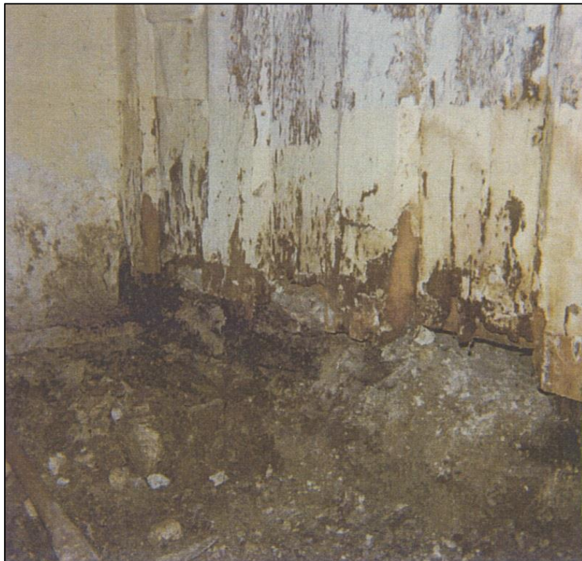
The bottom of the plank and muntin screen had rotted.
