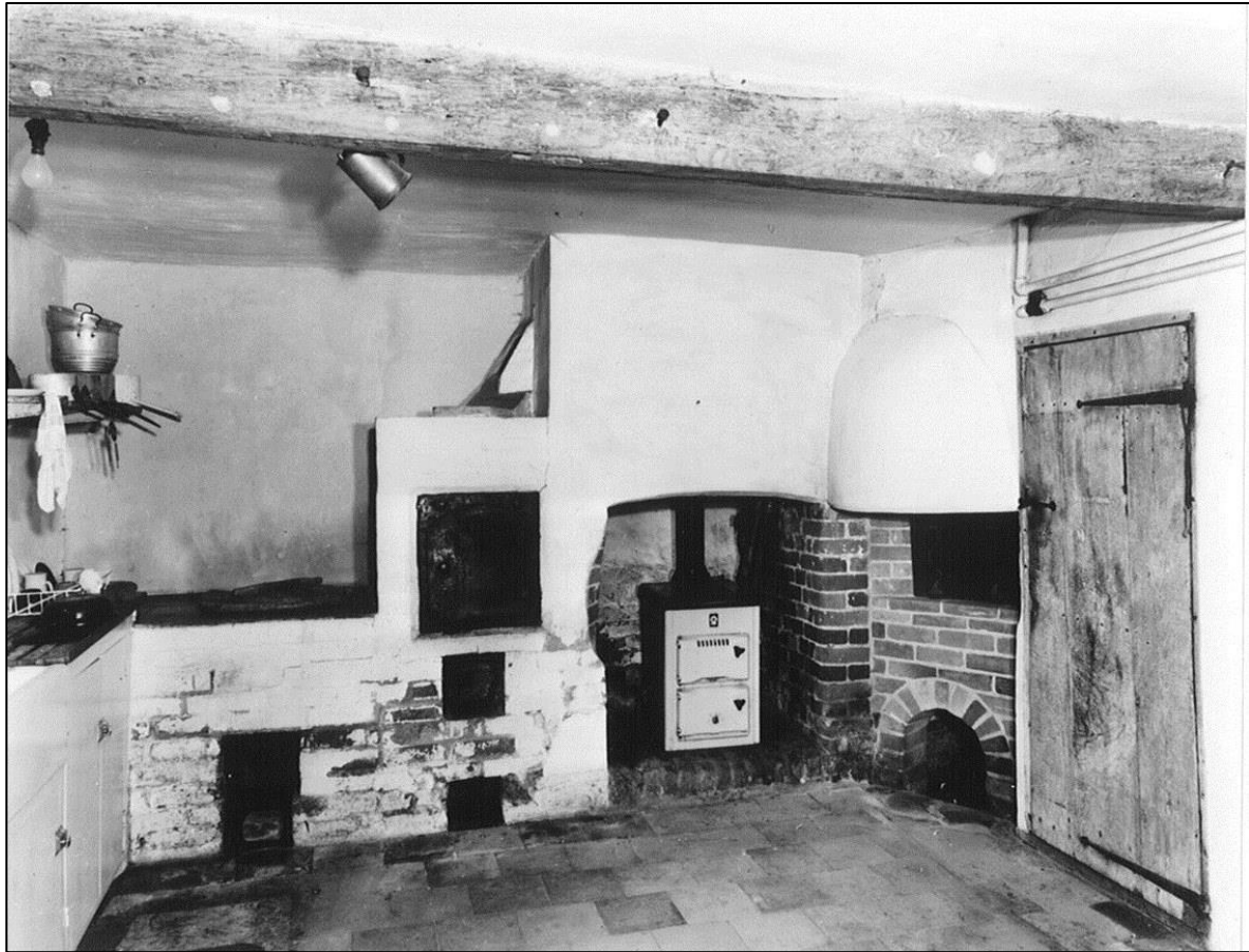
The kitchen as it was in 1979. A lot of damp was coming through the chimney wall.
