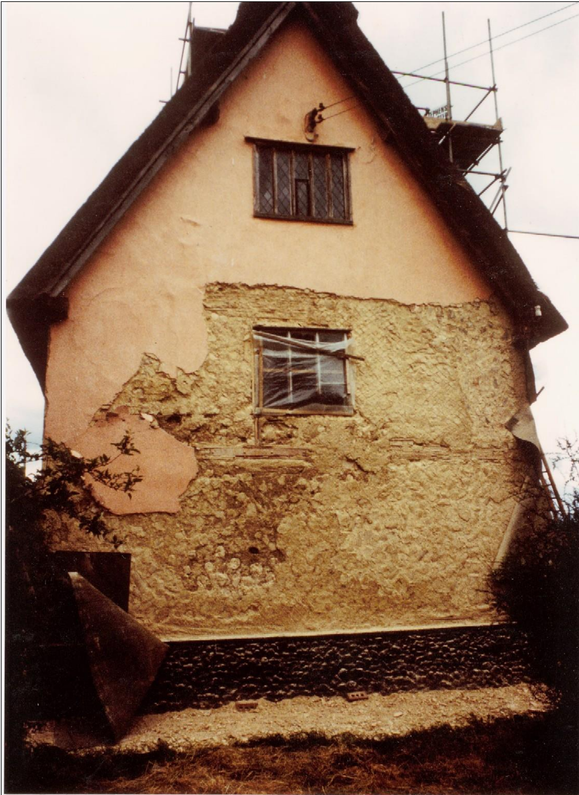
A bulge in the wall at the east end had caused the plaster to crack more than elsewhere so that it no longer formed a secure base for the coating of limewash.
