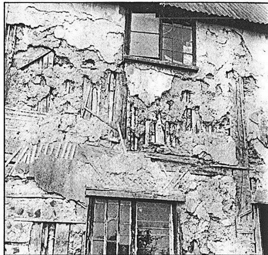
Exterior wall before repair.
