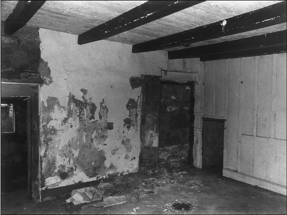
The door into the yard had been blocked but its frame was still intact. All that was needed was a new door. The wooden partition dates from the building of the house c. 1800. The floor once made up of old mill-stones, on top of which concrete had been laid.
