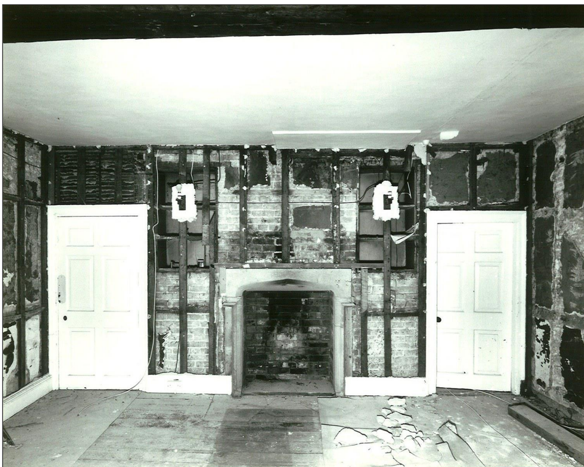
The North wall after hardboard was stripped off the walls and the passage partition was taken down.
