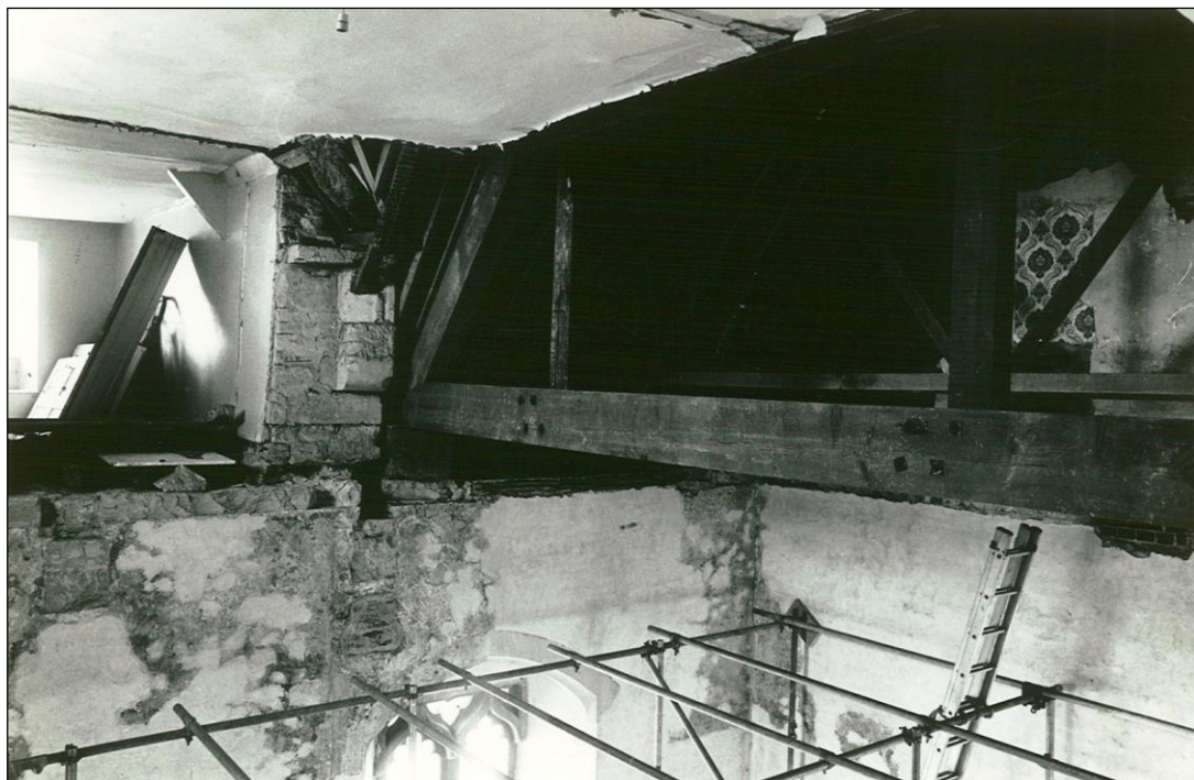
The tie beam over the King's Room, inserted in 1979, which had to be raised to allow clearance for the ridge beam of the new ceiling.
