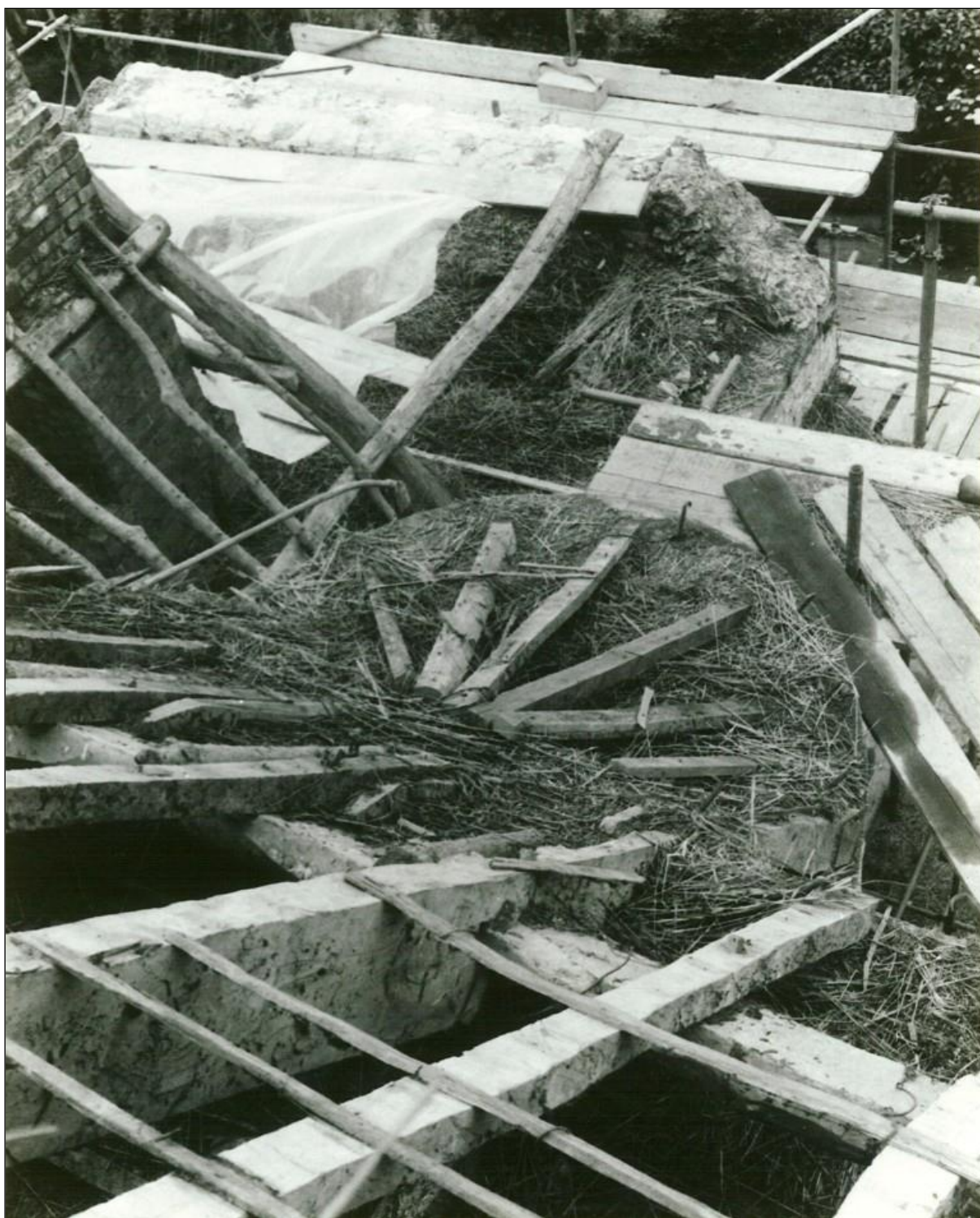
The old roof of the north turret and north west wing, after the thatch was stripped off in 1979
