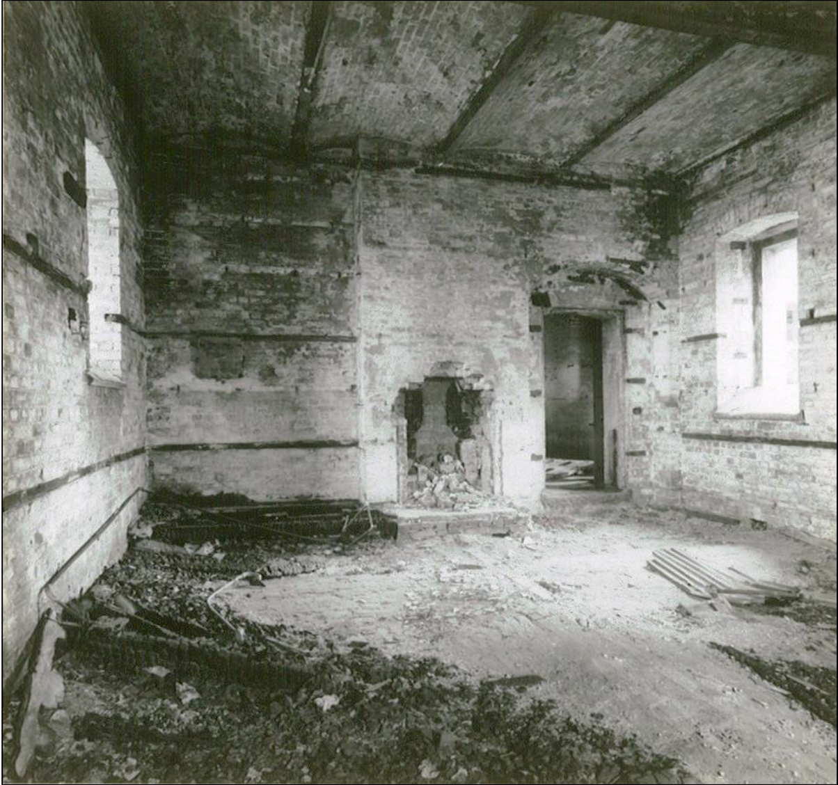
The north barrack, now the living room, with the charred remains of the floorboards.(NMR)
