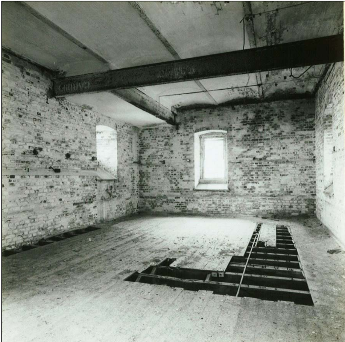
The west barrack, now subdivided into bedrooms and bathrooms. The concrete structure supporting the mount of one of the roof guns can be seen on the left, with a girder to give further strength. (NMR)
