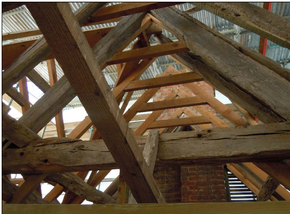
Repairs to the roof structure. The clasped purlin (left) is suggestive of an early (17 th -century) construction date. Unfortunately, the timbers were not suitable for tree ring dating.
