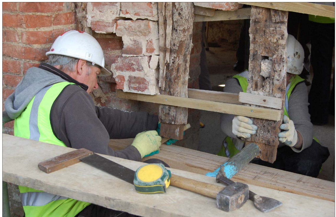
Top: the façade was stabilised and tied in using a tile-stitching technique. Below: repairs to the timber framing
