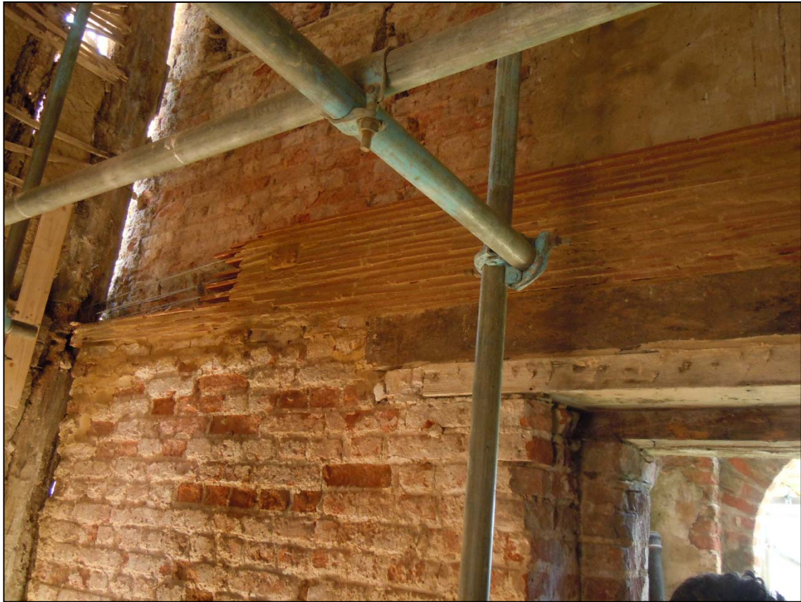
Top: the façade was stabilised and tied in using a tile-stitching technique. Below: repairs to the timber framing
