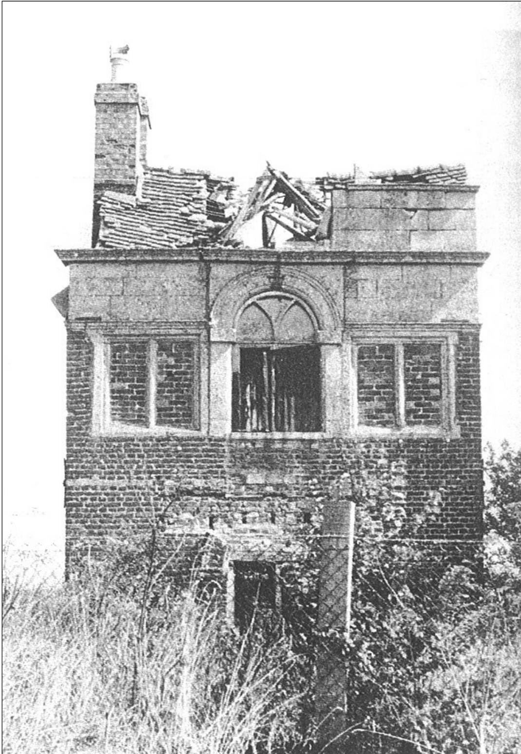
The Warren House at in 1985, at its lowest ebb, before the repairs carried out by the Boots Pension Fund. ( Ancient Monument Society's Transactions , 1985 Vol 29)
