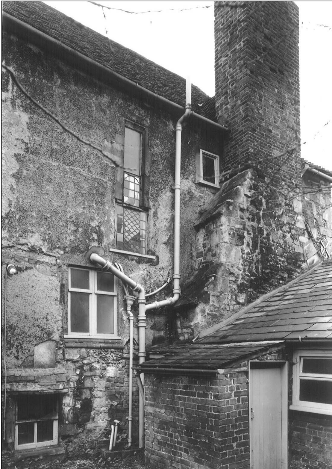
The north end, with its great chimney, has much medieval masonry, and some blocked medieval openings, as well as the jambs and lintel of the tall window which lit the chamber above the kitchen. The rendering was removed, and the wall, which was bulging under the weight of another chimney, was secured. Some original openings were restored, and later ones blocked to rationalise the arrangement. The low building was added in the 19 th century (NMR).
