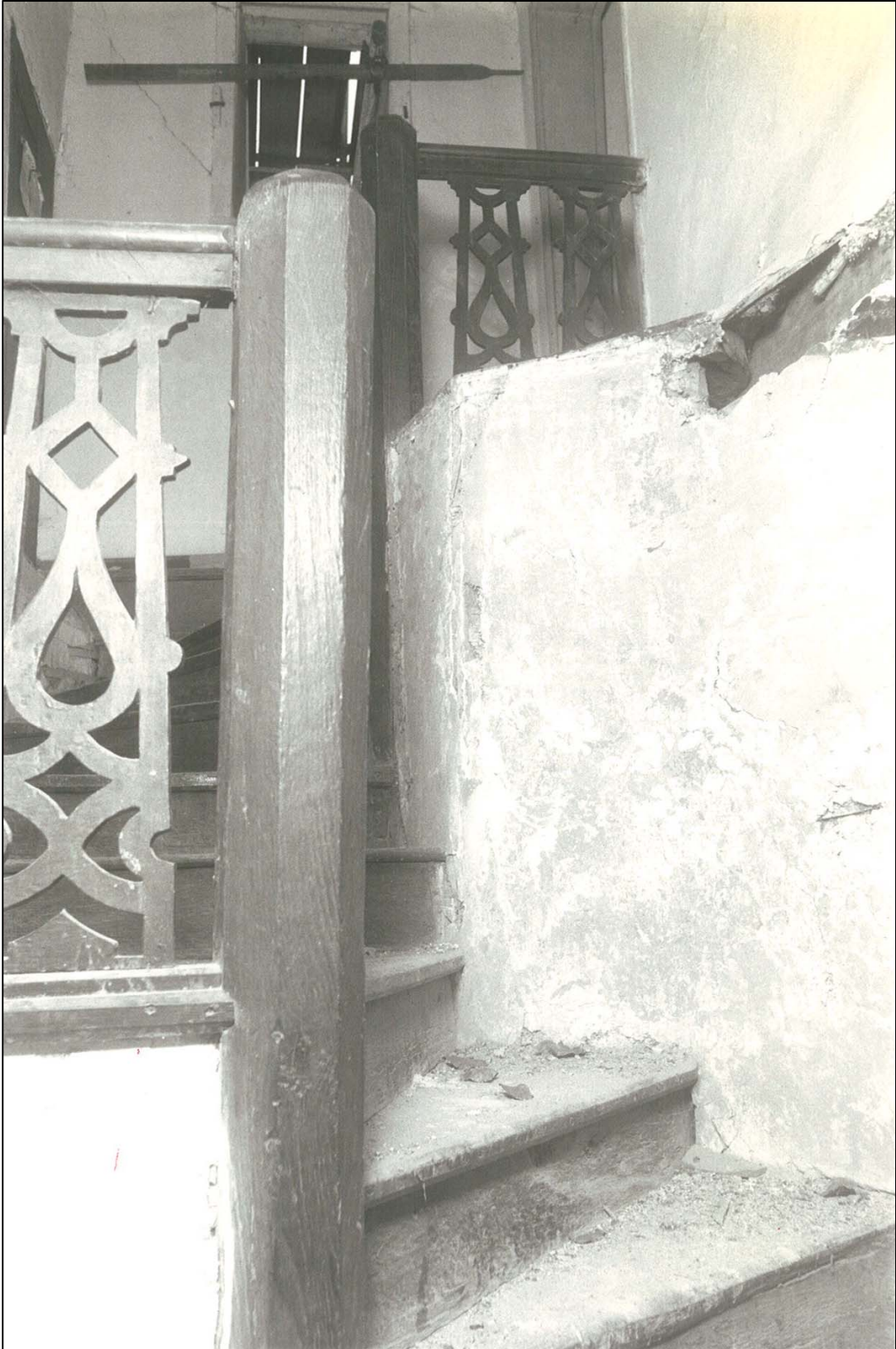
The 17th-century stairs leading up to the Landmark flat. The balustrades, of the same date, are similar to the altar rails in Great Durnford Church. The treads needed reinforcement, but otherwise they have just been rubbed down and waxed.
