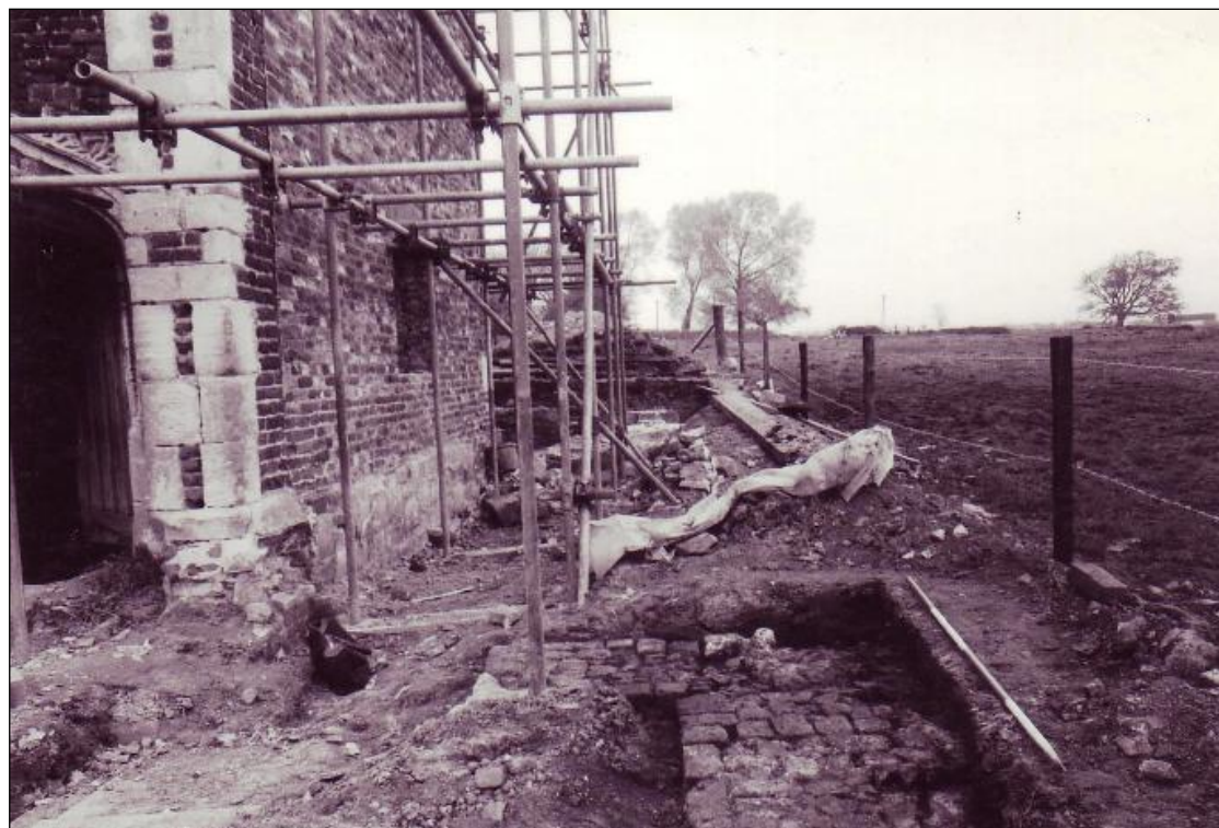
The foreground shows a brick footing for the demolished wing of the mansion, partly re-using Abbey stone.
