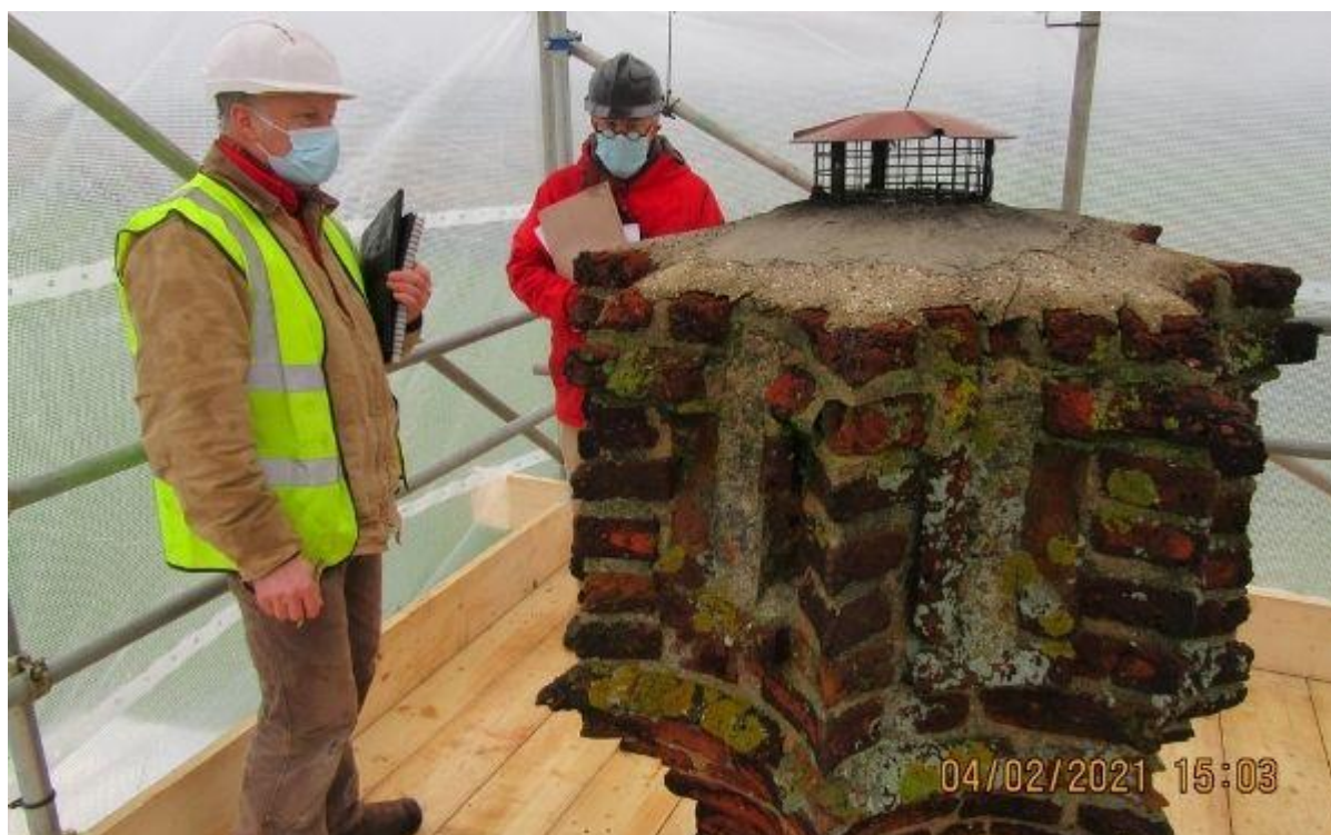
Conservation architect Philip Orchard (left), and Landmark surveyor Stephen Donelan inspect the weathered chimney prior to its repair. It was highly sophisticated work – then and now.
