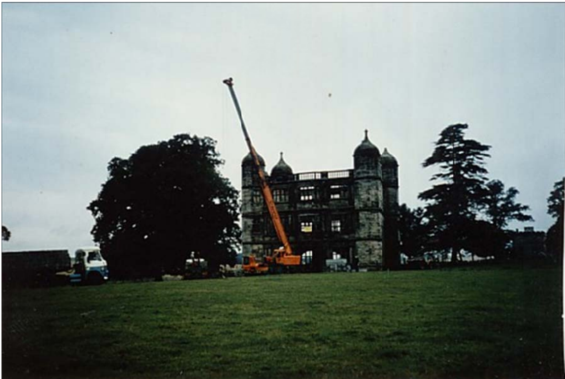
A crane was used to lower materials into the building, to avoid having to use the narrow staircases.
