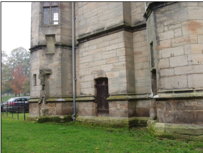
Examples of anomalies at Tixall: top blocked doorways on ground and first floors on the east elevation, with masonry scars where earlier walls were keyed into the gatehouse; bottom, blocked doorway in the NW turret.
