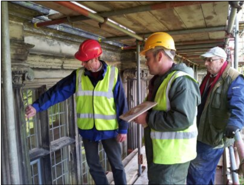
Landmark's surveyor for the West Midlands, Richard Burton, discussing the work with the masons from Midland Conservation.
