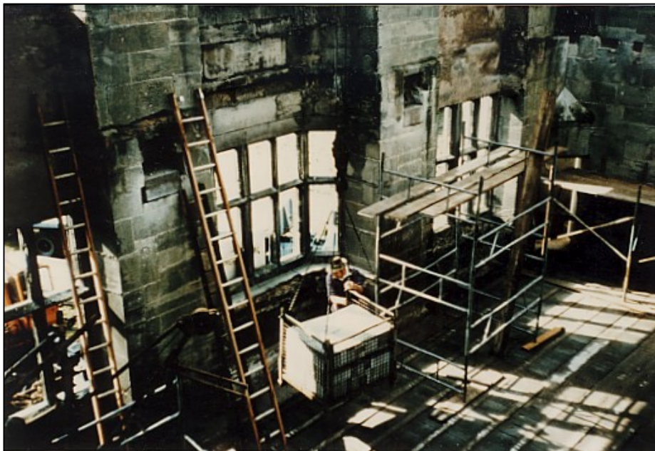
The first floor is complete, but materials can still be lowered by crane through the open roof and upper floor.
