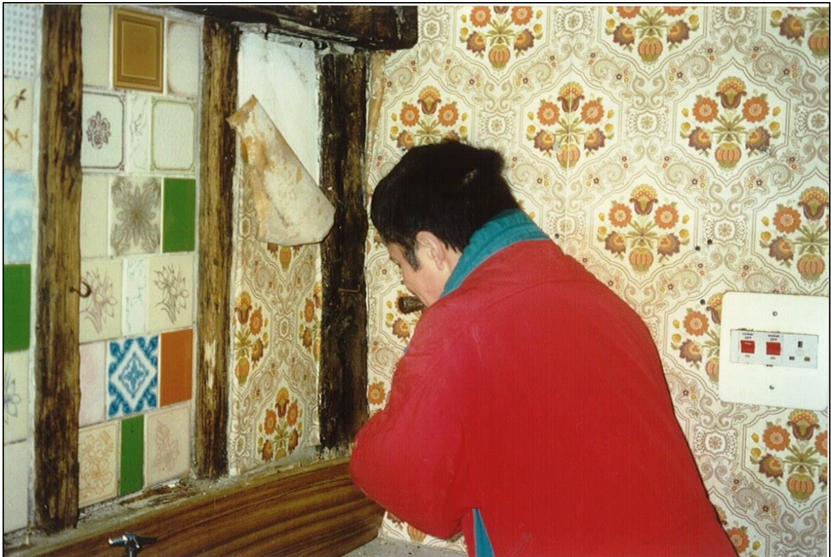
Architect Philip Orchard investigating what remains of the blocked 15 th century window.
