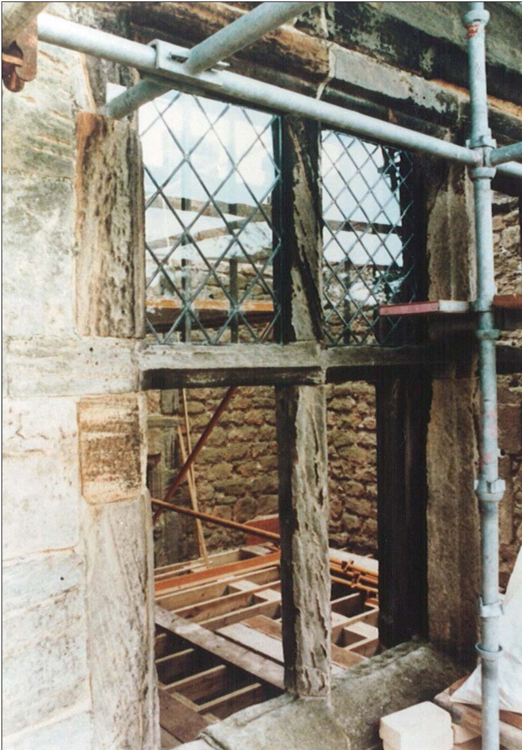
Different patterns of glazing, and sizes of panes, were looked at in the building before a final decision was made (above and overleaf).
