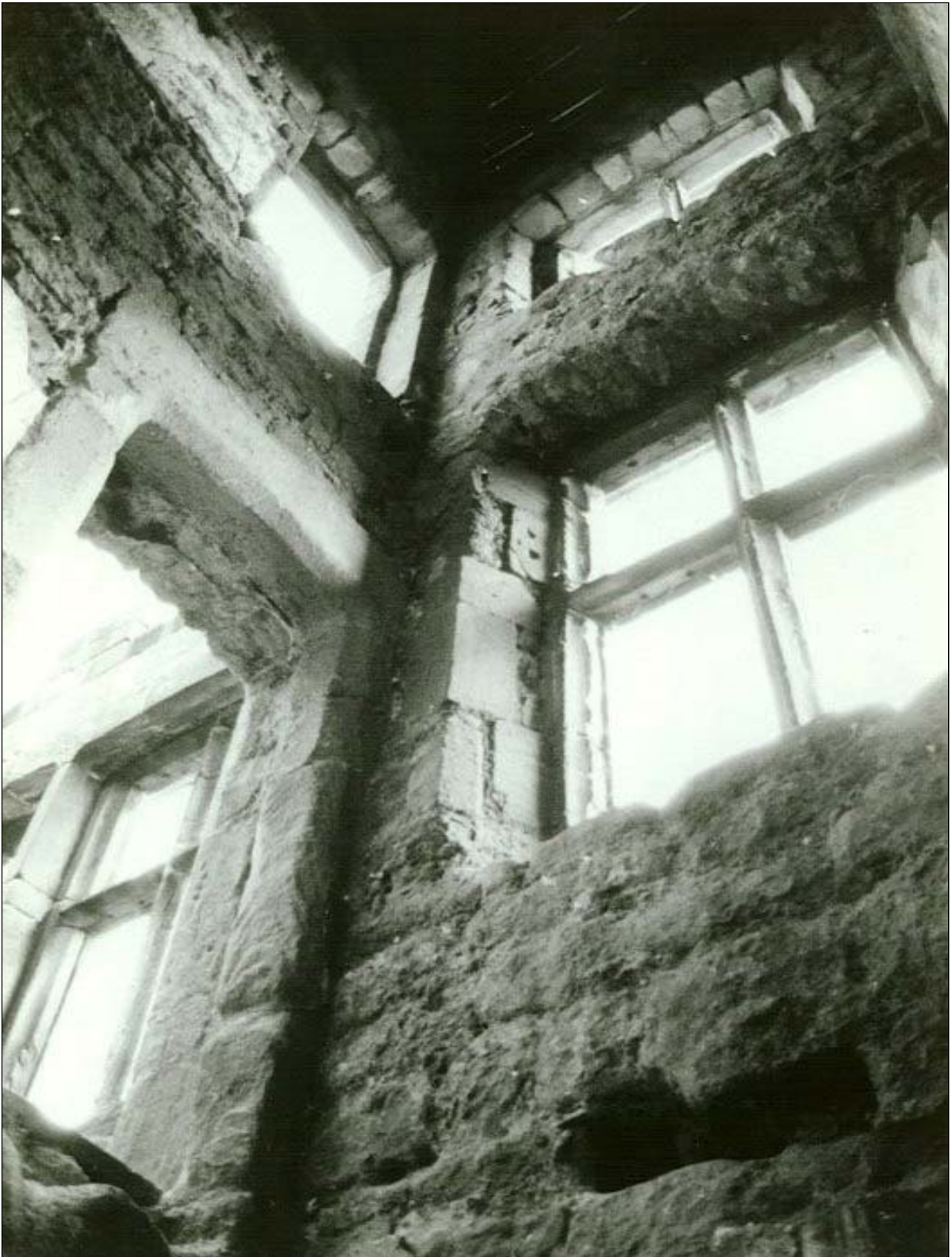
Open window, before repair.
