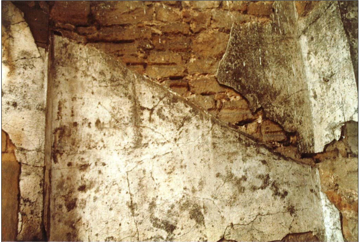
The line of the original staircase showed in the plaster of the stair turret.
