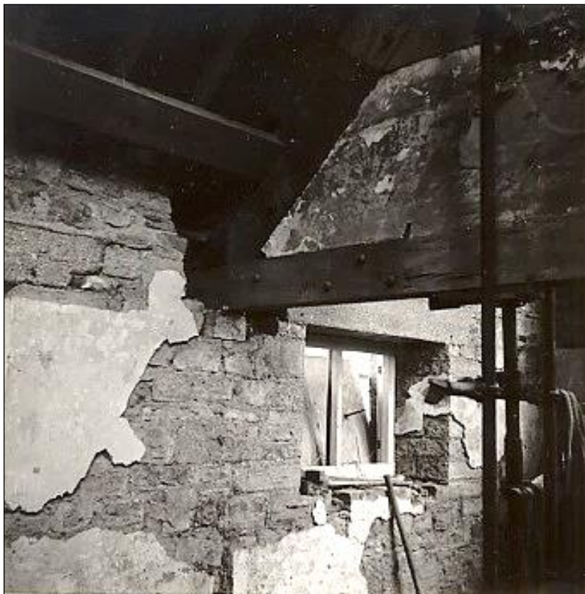
17th-century wattle and daub survived in the area of the closed truss.
