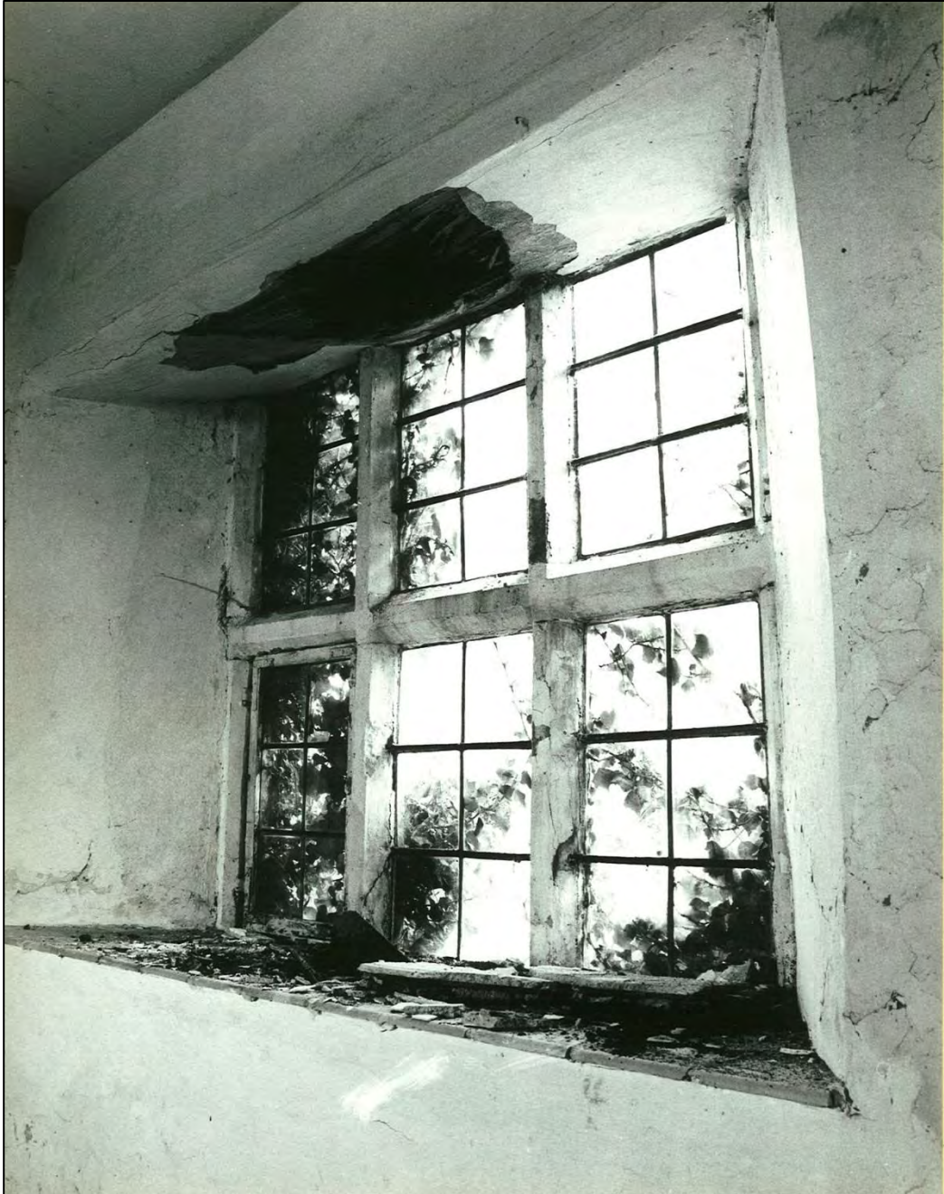
The back window on the first floor. The building was suffering badly from damp, mainly caused by decayed cement render on the walls.
