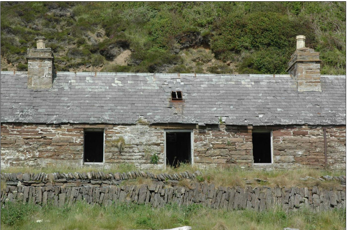
The Shore Cottages before repair.
