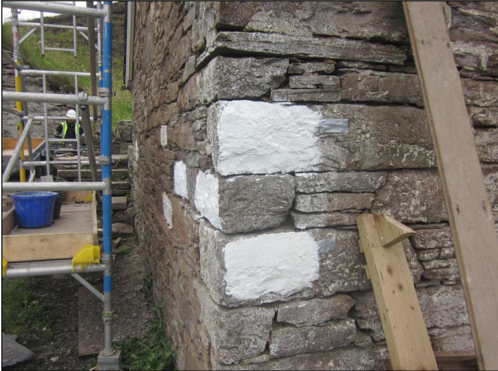
Limewash trials. Note too the quality of the masonry and carefully laid courses. The cottages were clearly built by skilled professional masons.
