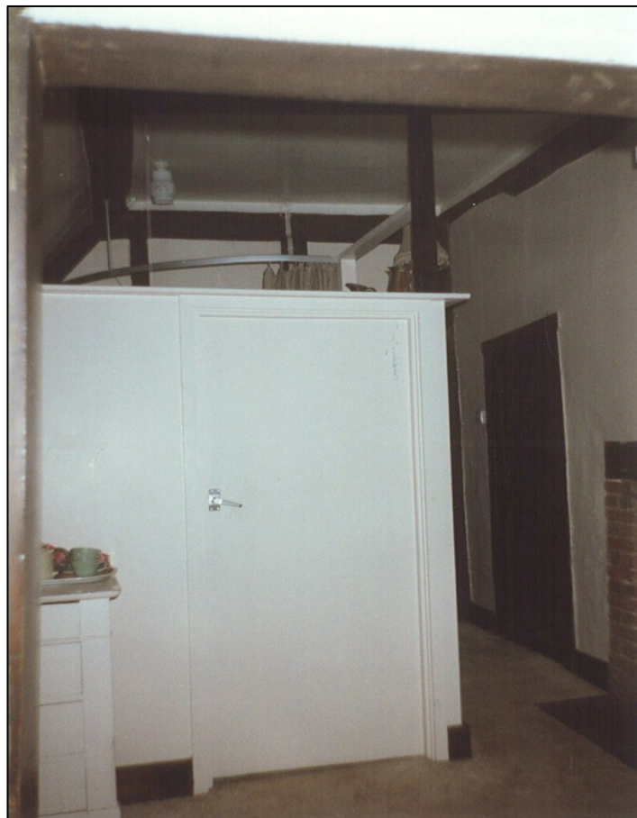
This bathroom 'pod' was removed from the what is now a single bedroom.
