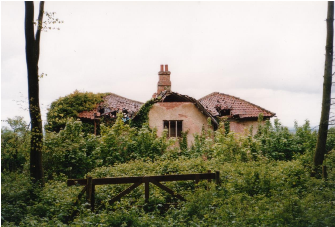
South elevation before restoration, all render lost. The scraps of wood bottom right are the remnants of the giant trunks that once framed the door on this elevation.
