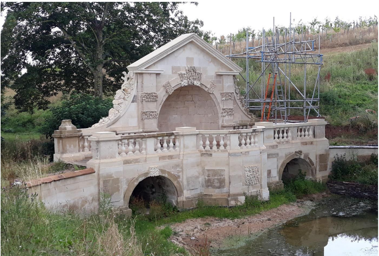
The Bath Stone Bridge in 2018, restoration almost complete. Most of the screen has been skilfully re-carved, matching and interpreting the original fabric.
