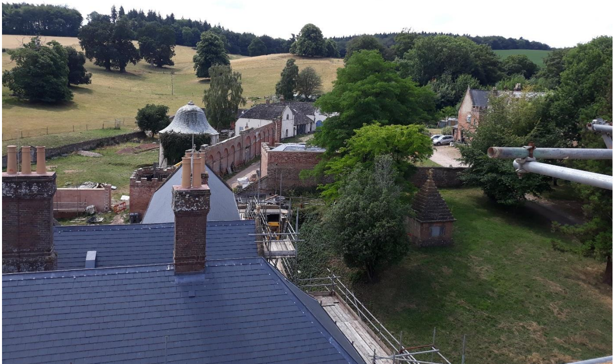
View from the roof of Halswell House in 2018, with the repairs to the Tudor buildings well underway. Robin Hood's Hut is behind the second large oak at the left.
