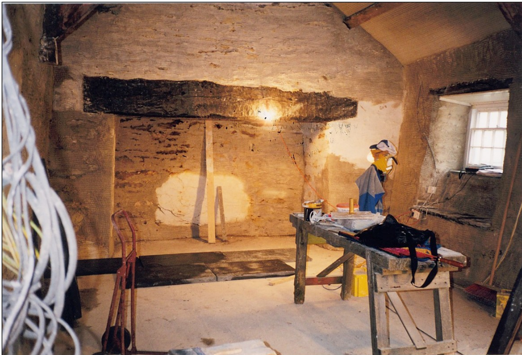
The scratch coat of lime plaster now on the walls, it was time to think about laying out the floor.
