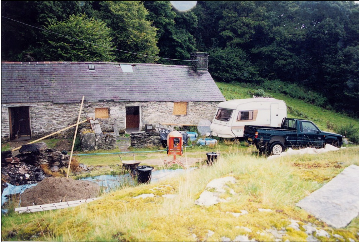
The exterior during the early stages, with the front skylights and overhead power cables still apparent.
