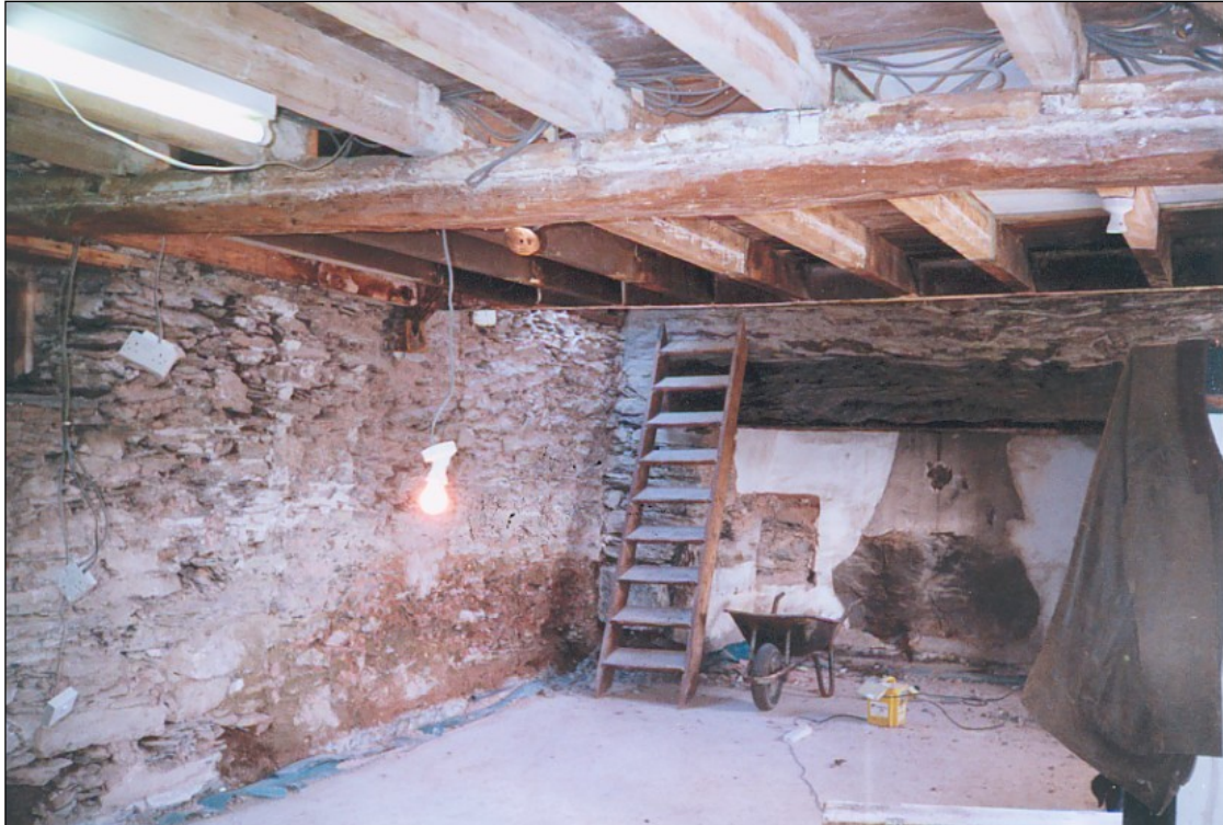
Early stages, with the walls stripped of modern plaster and the modern extension of the croglofft to the point where the second tie beam was.
