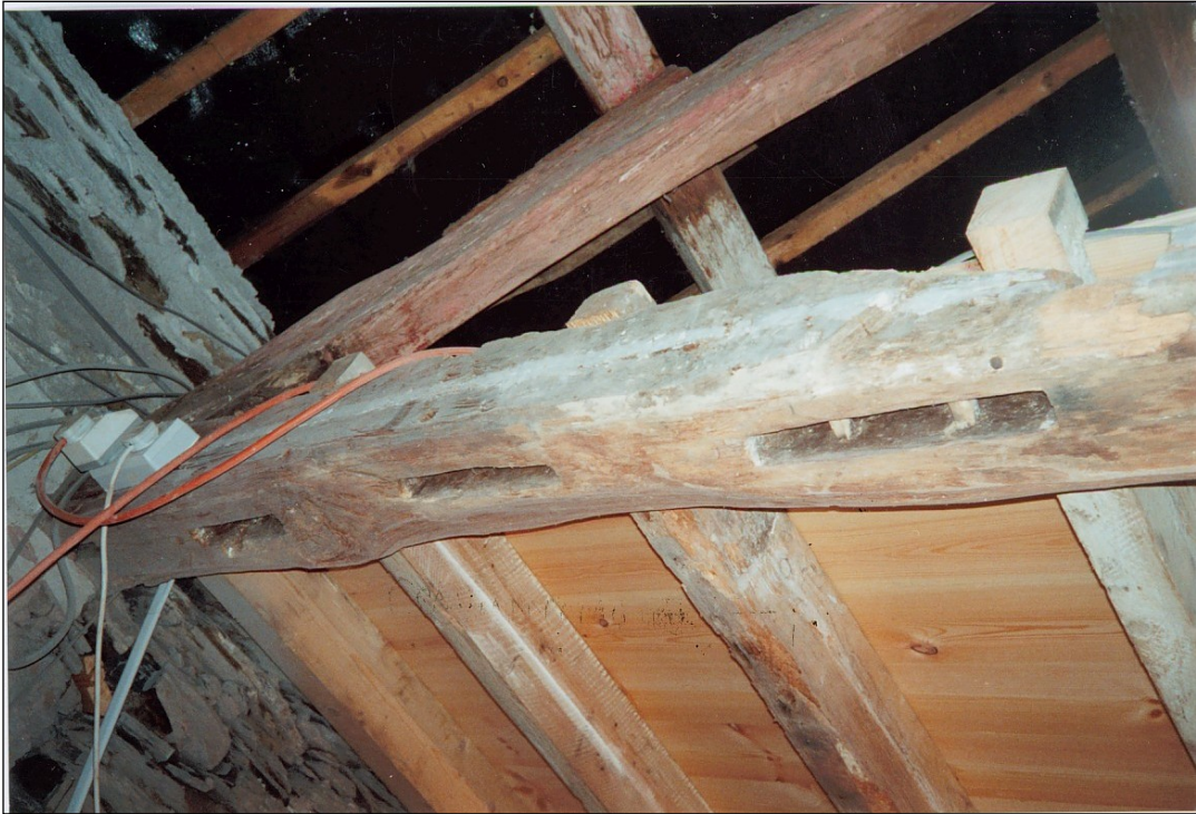
The remaining tie beam, showing the mortices for the former plank-and-post partition and the groove where a ladder may have rested. The joists for the new bedroom ceiling rest in the original notches.
