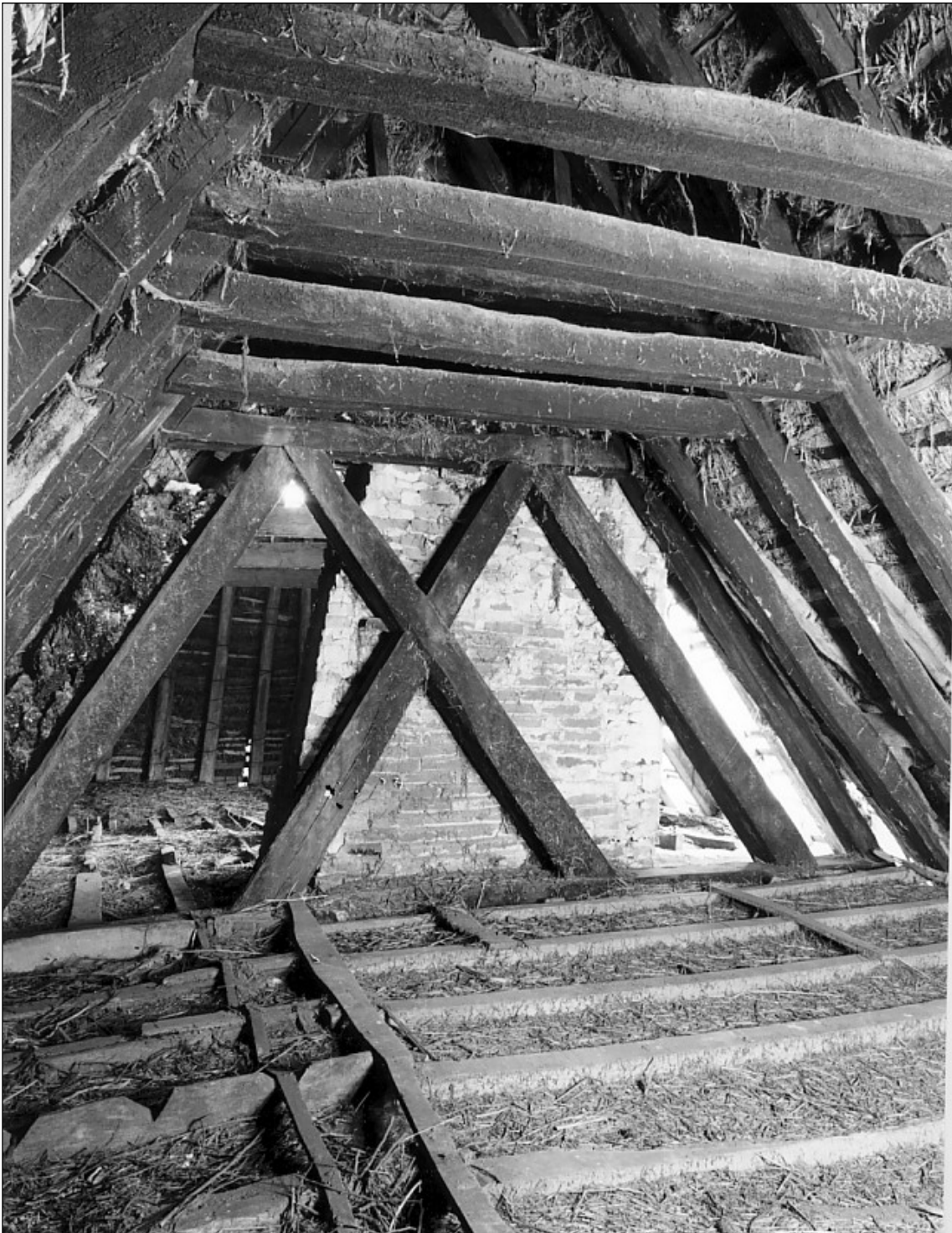
The High End truss before the removal of the first floor and chimney stack.
