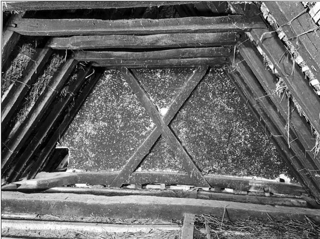
Late medieval smoke blackened plaster in low end. Closed truss found in roof space above first floor ceiling.
