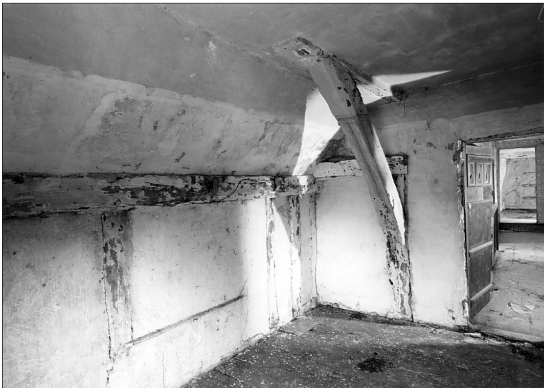
North side of north-east arcade post, and arcade plate, in north east first floor room.
