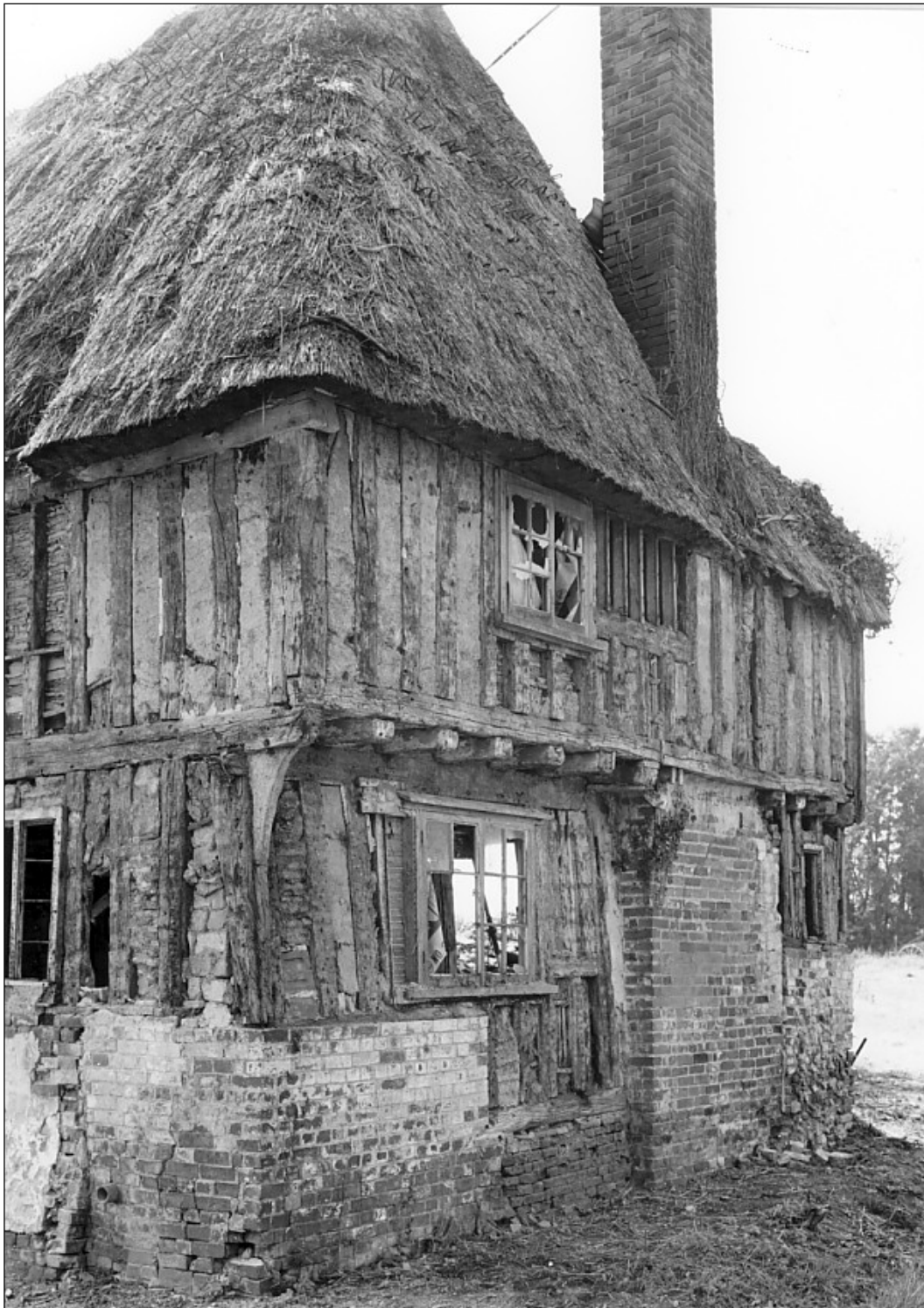
The jettied north end, after plaster was stripped off in 1970. A window with original mullions emerged on the first floor.
