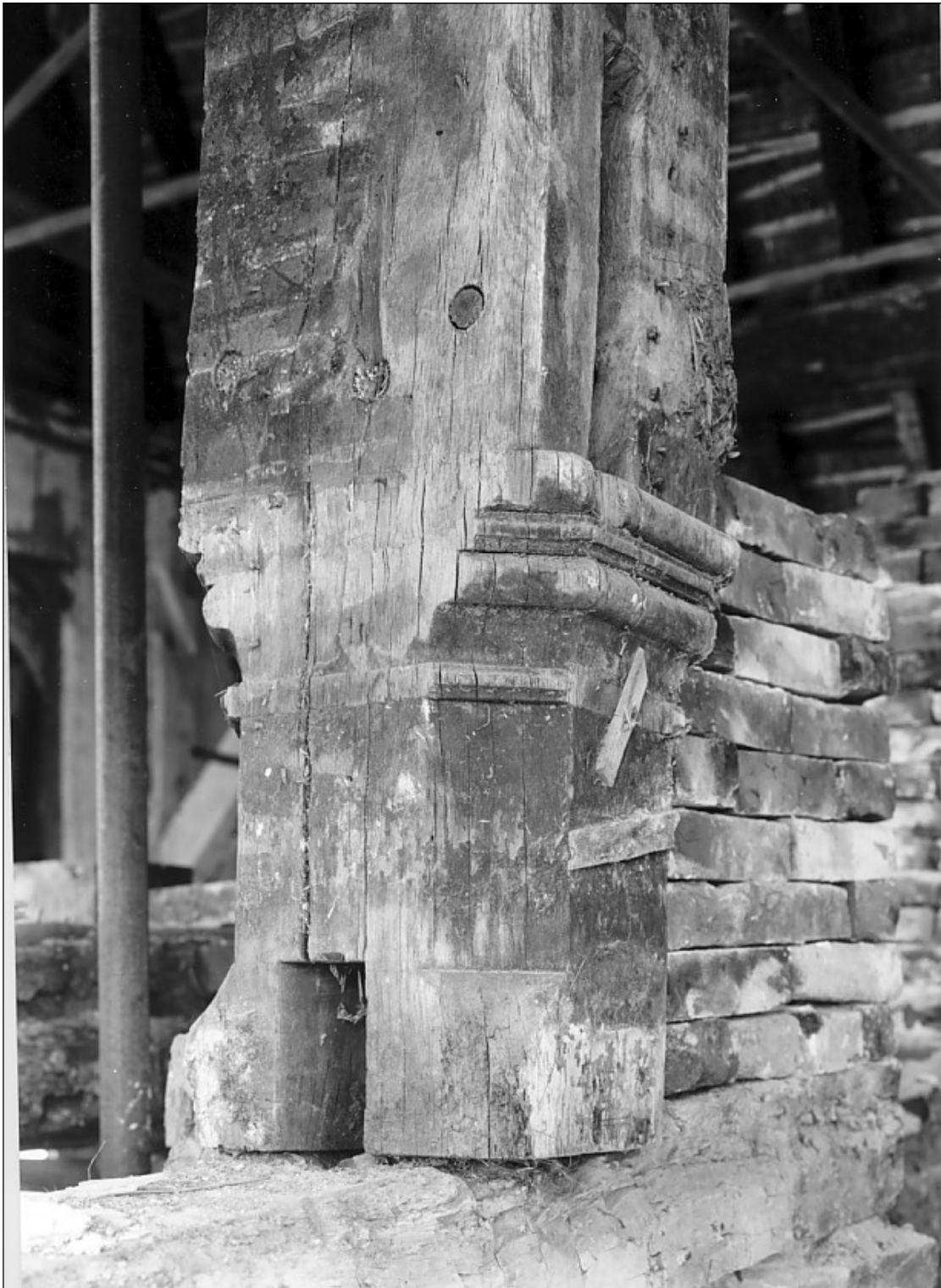
The South West arcade post cut away when the chimney stack was inserted.
