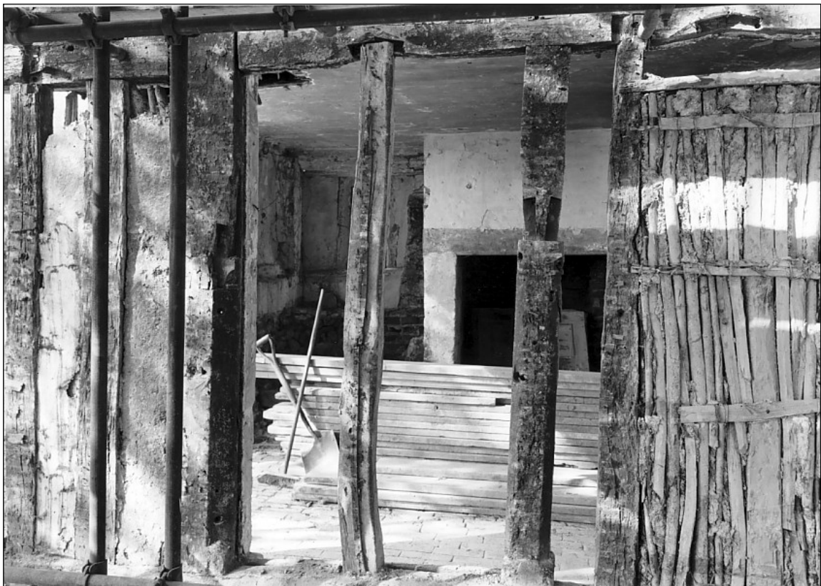
Close up of arcade, in which the mortices for the arcade pieces can be seen.
