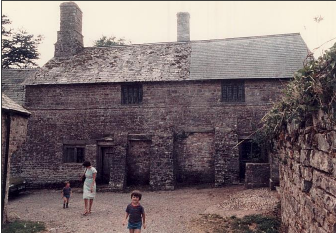
The east elevation. The roof repairs to the northern half, after a tree fell on the building in the 1960s, are clearly visible.
