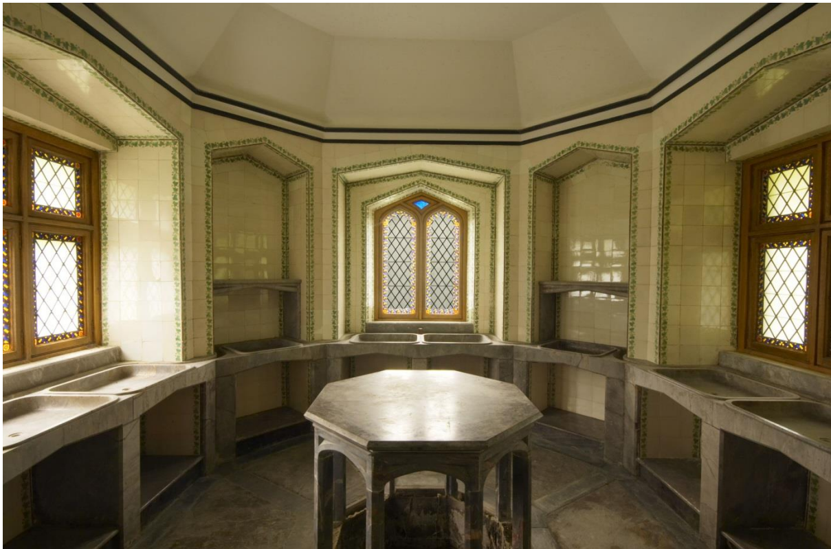
Inside the Endsleigh Dairy, before and after restoration. Note the ivy leaf pattern tiles edging the windows and alcoves.
