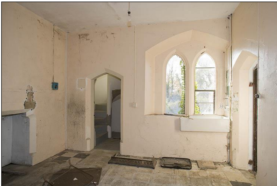
Looking south across the former kitchen before works began. The hearth for the range is on the left.
