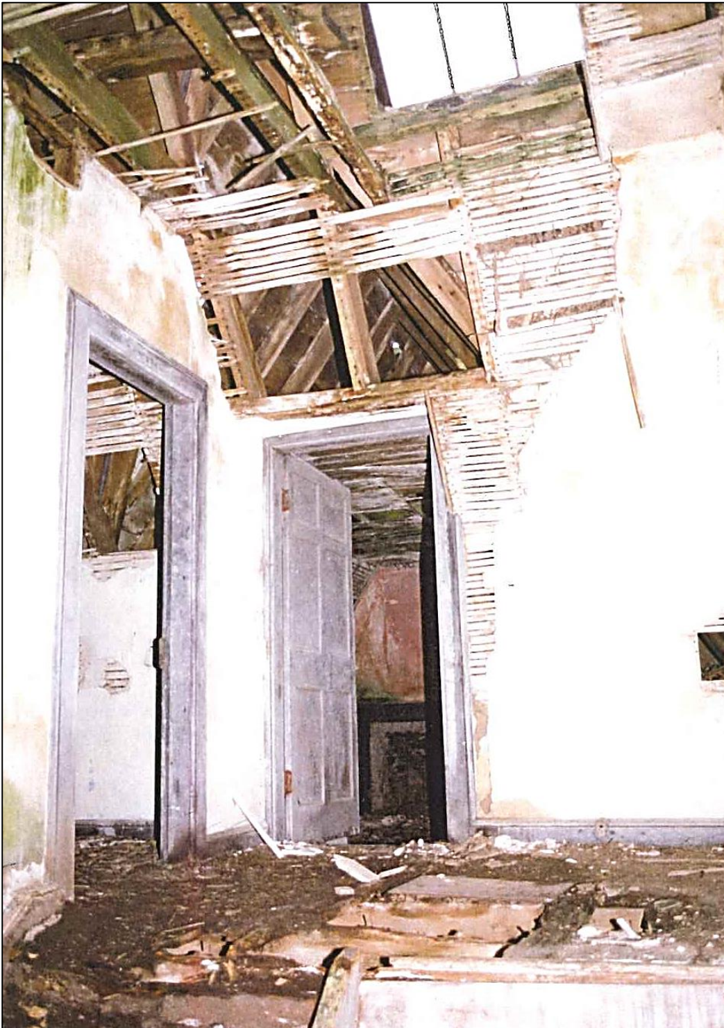
The top of the Victorian staircase and the first floor landing. The floor boards were rotten and were replaced with second hand pitch pine from the Midlands.
