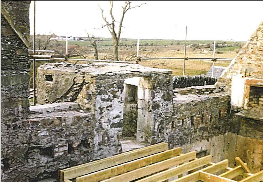
The top of the spiral staircase without its roof, and the first floor ceiling being replaced at its original level; it had been raised in the 19th century.
