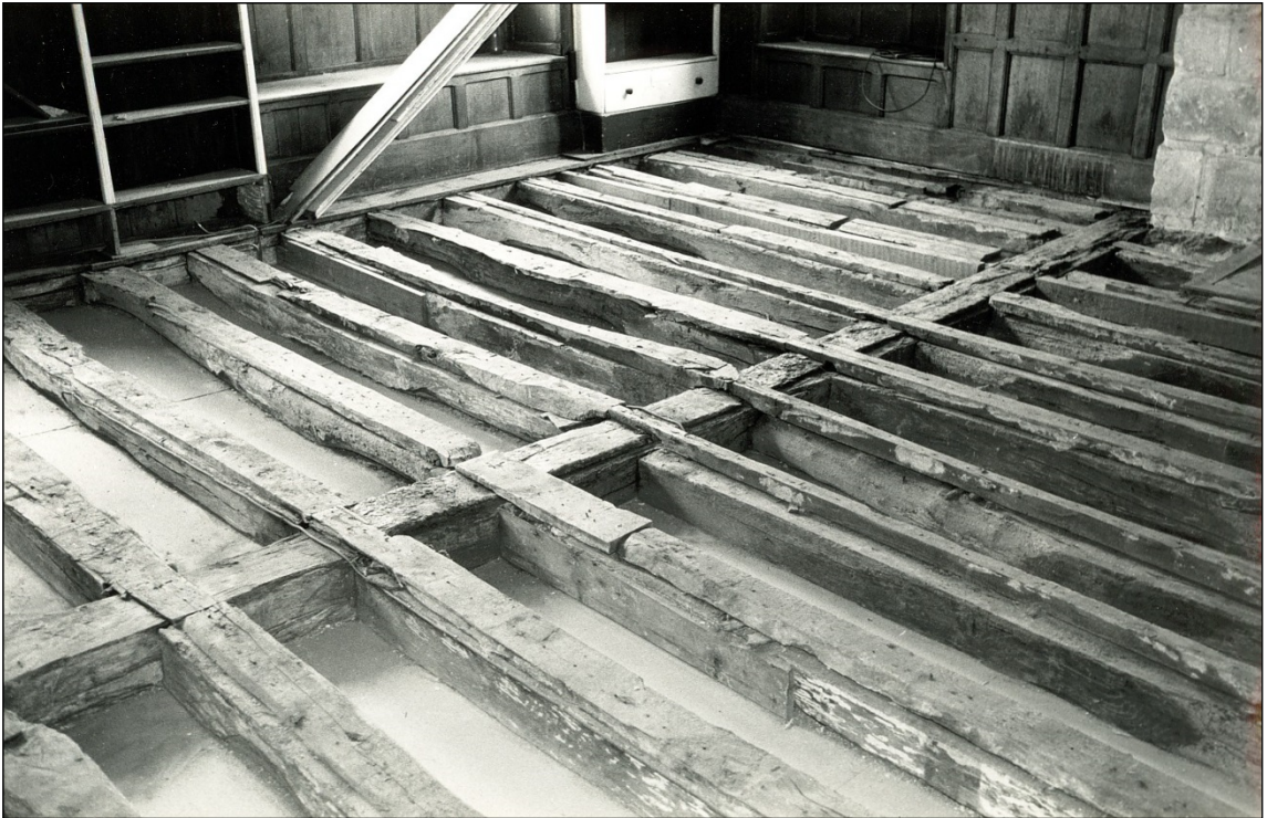
The medieval floor joists in the study, on the first floor of the South Block
