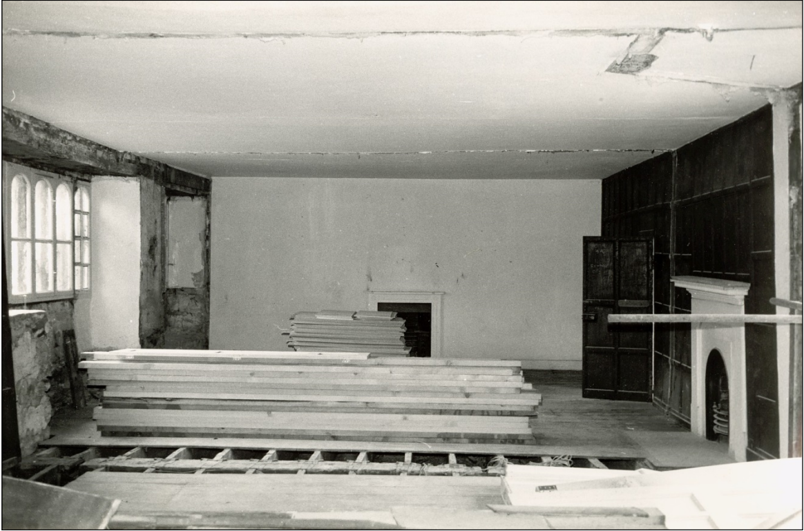
The end frame of the east wing added c. 1425. On the right an earlier brace of the main block's original timber frame can be seen
