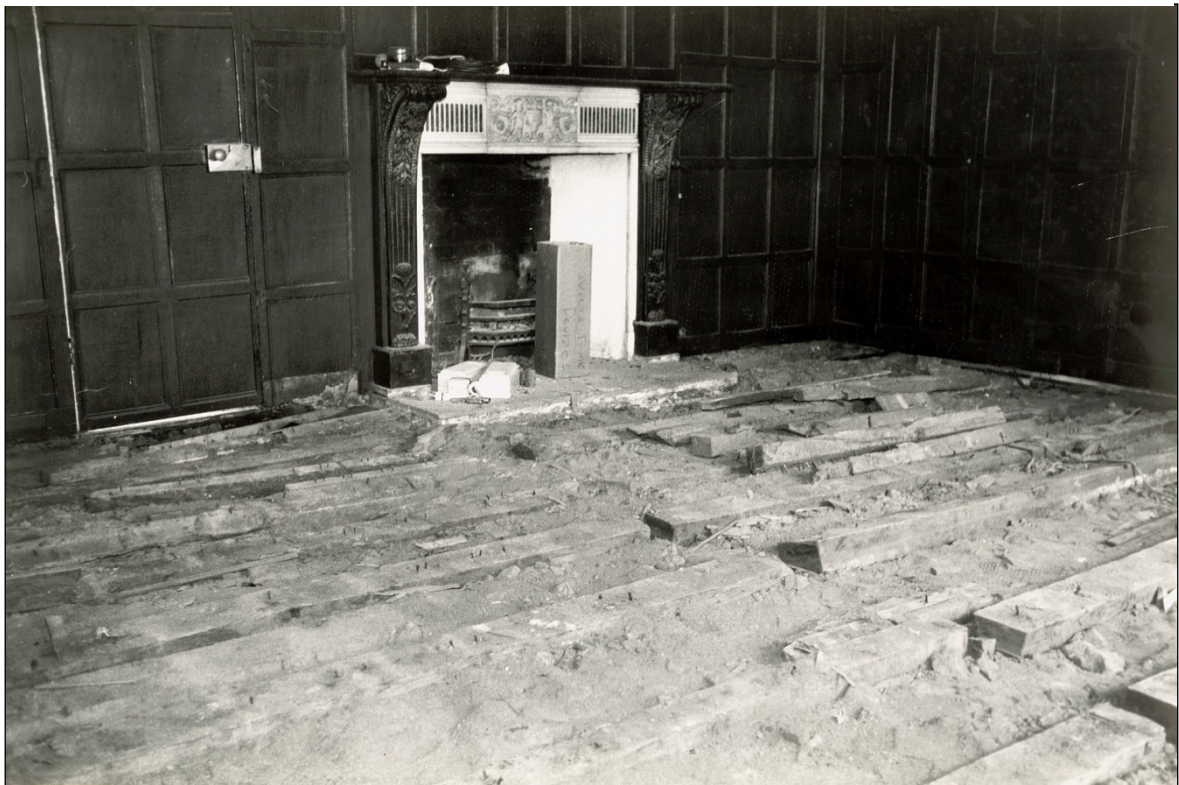
The Tudor joists, lying directly on the ground in the drawing room
