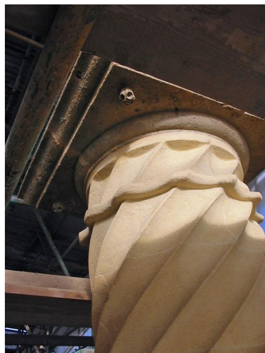
Original stone carving detail of the small gotti beneath the square plinths of the chimneys.
