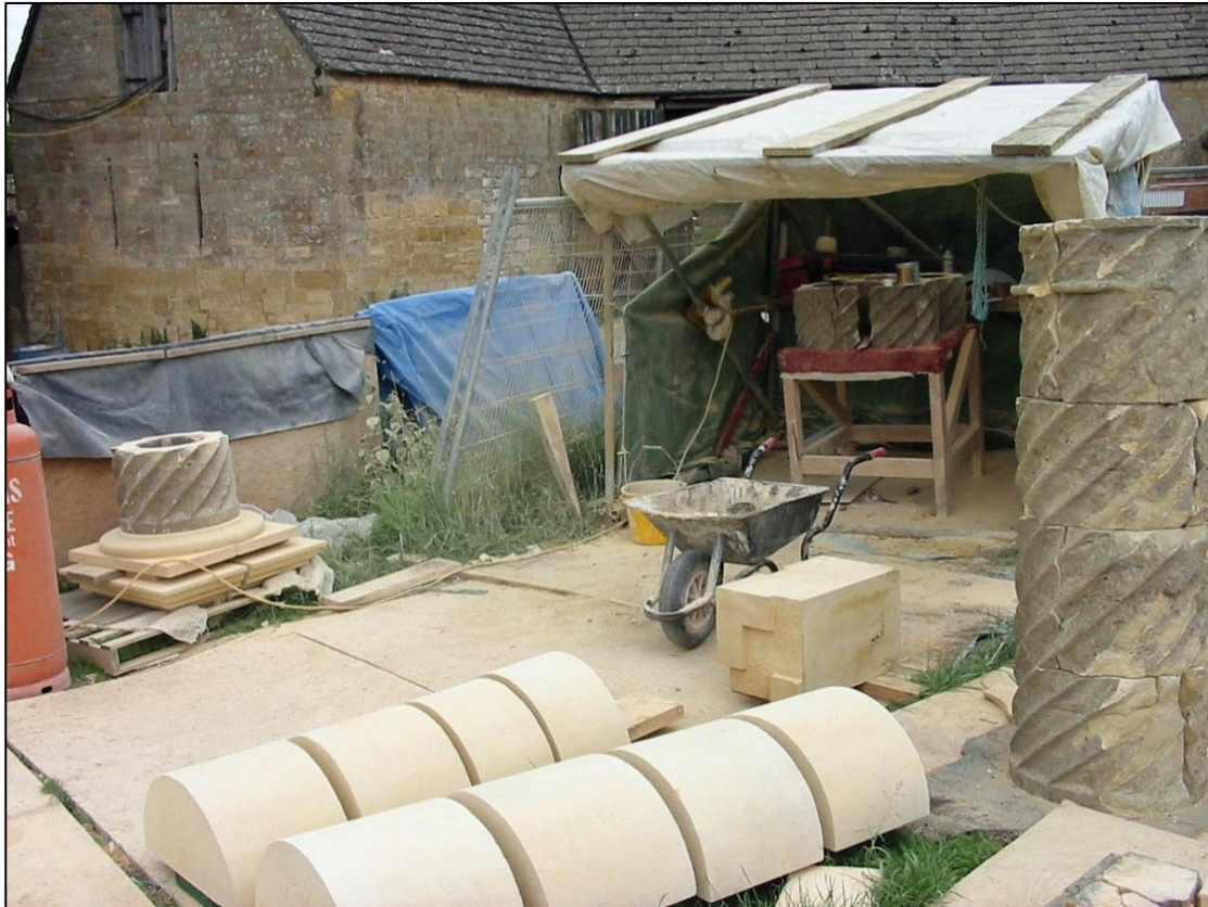
Two new chimneys were built on site in a traditional stonemason's bankers' shed, June 2002.
