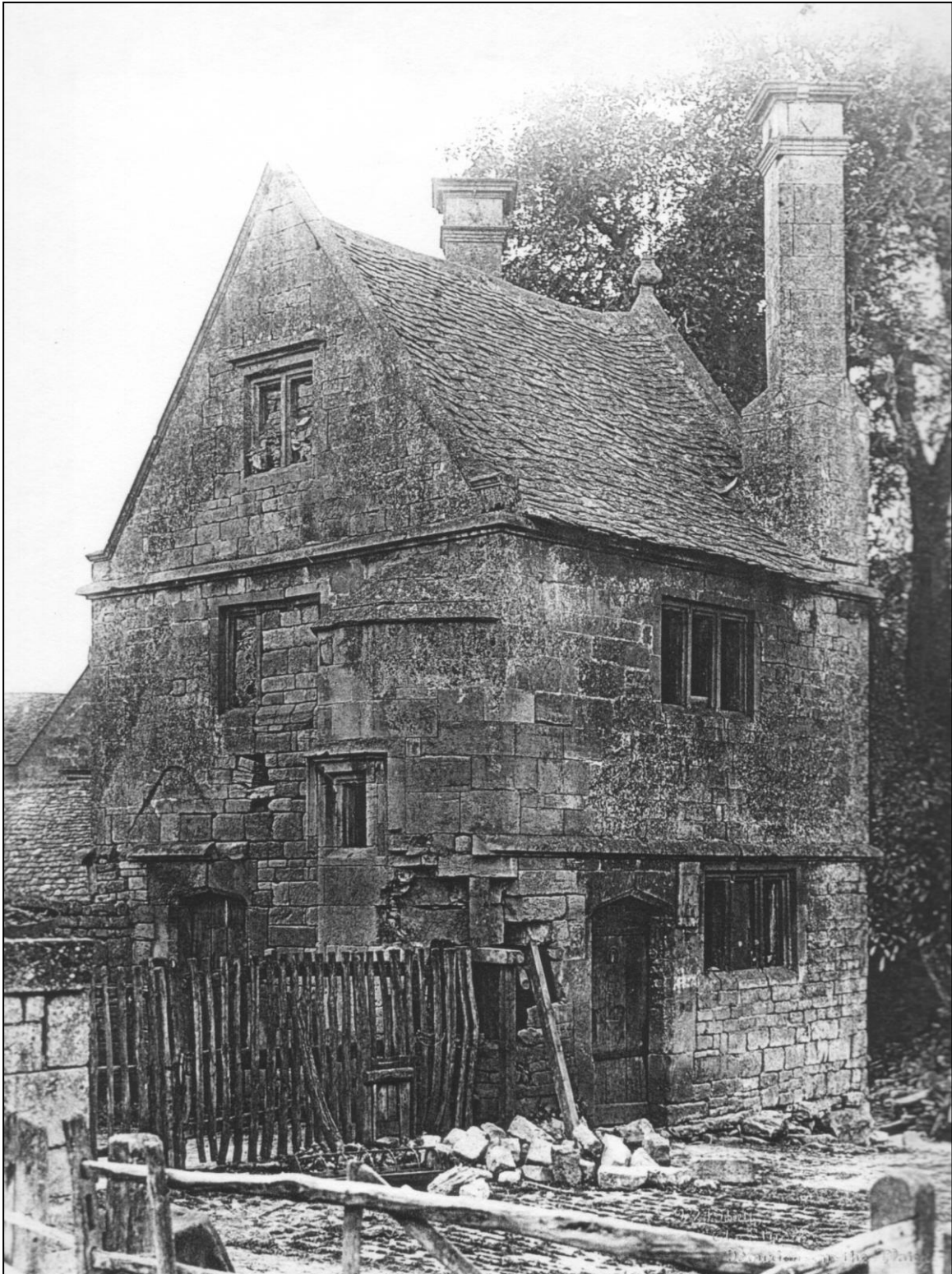
The Almonry before its repair in 1929. The removal of the lean-to (see Fig 29) has made the dangerous state of the stair turret alarmingly clear.
