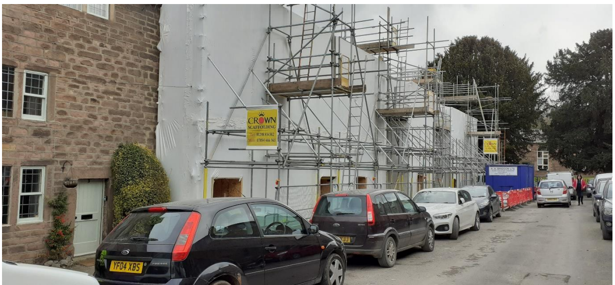
Half the north side of the street had to be swathed in scaffolding from October to March.
