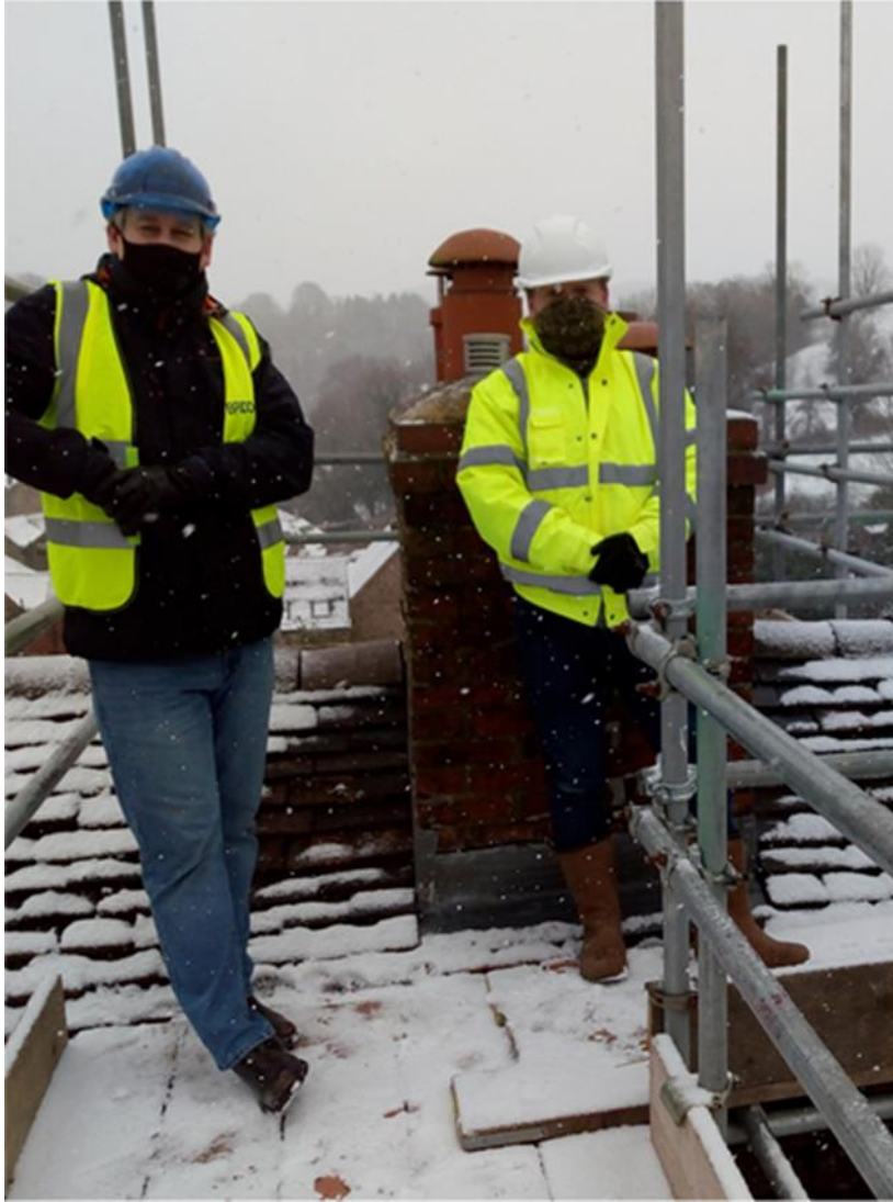
Outside works meant that the project could continue despite lockdown, but the winter of 2020/21 saw some very cold conditions, as here in February 2021 when film maker Mark Todd (left) visited to film the works for Historic England.
