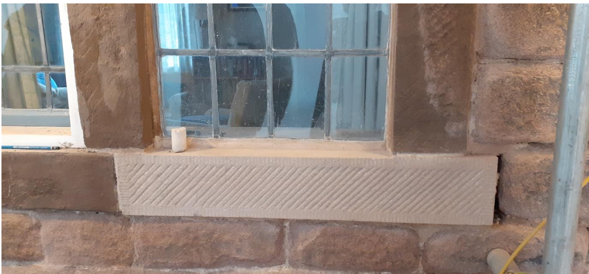
Replaced window sill, with plastic repairs visible as the as yet darker areas in the eroded jambs just above the sill. As they dry, they will be hardly visible.
