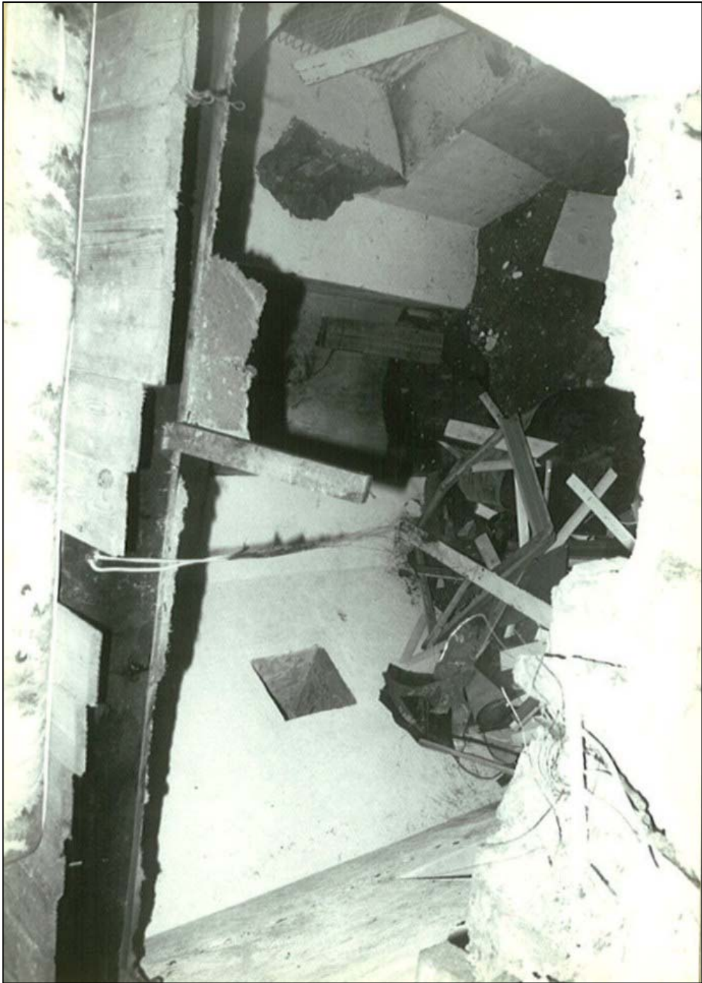
Looking through the hole in the first floor towards the ground floor
