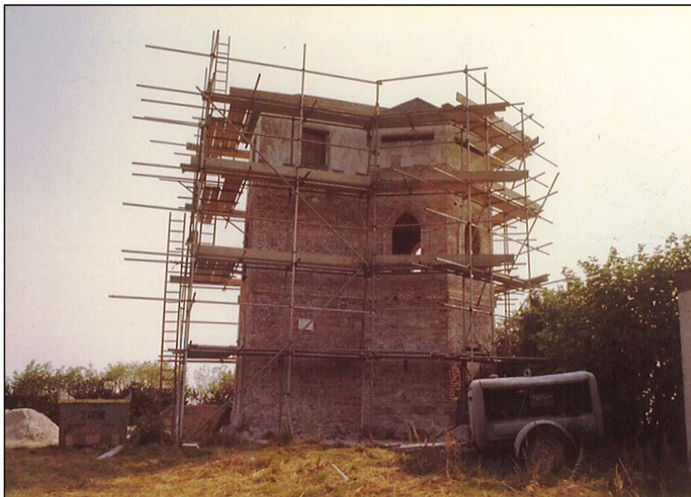
1983. The crenellations of the original building can just be seen behind the scaffolding.
