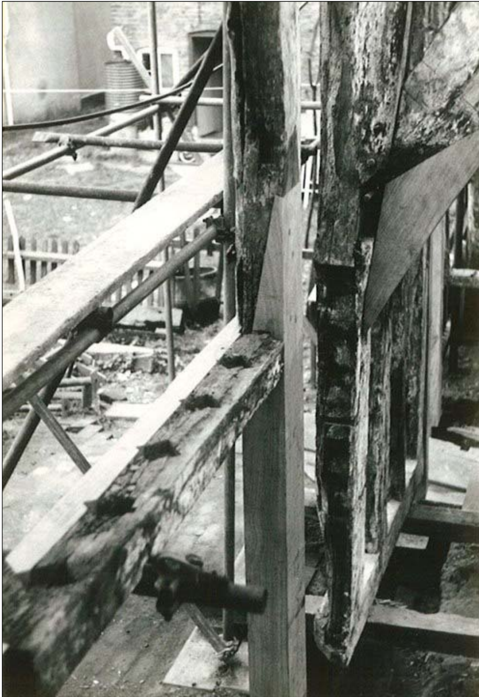
The repaired rear wall seen from a high level within. As much of the original frame was kept as was possible, and the repairs are easily distinguishable to avoid any confusion with original fabric. In the foreground are the sockets for window mullions discovered for the great window on the back wall.
