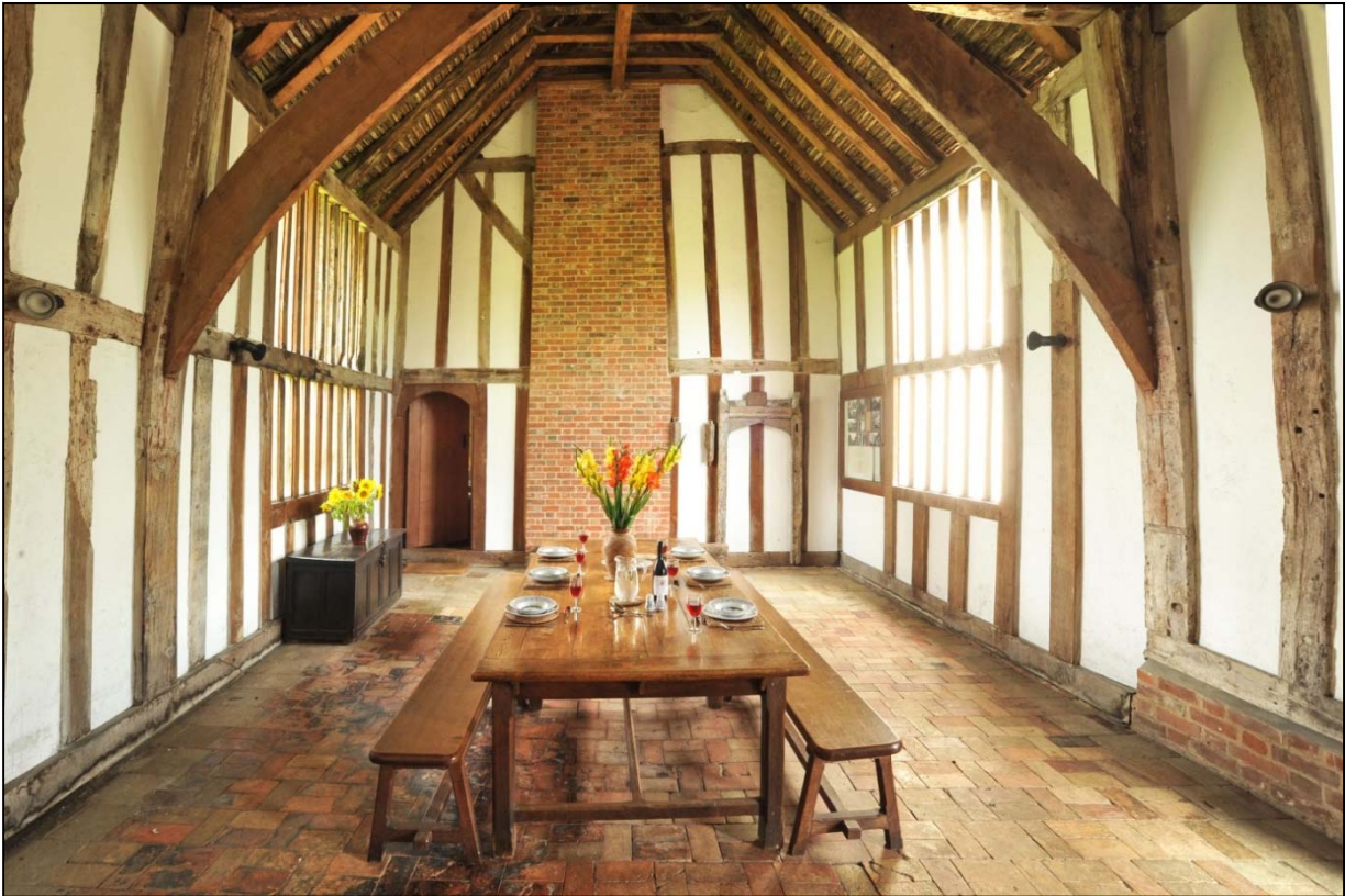
The hall at New Inn before the 2013 refurbishment. Note the underside of the clay roof tiles open between battens between the rafters. The brick panel indicates where the lost inserted stack cut through the timber frame – and, like it, helps support the building.
