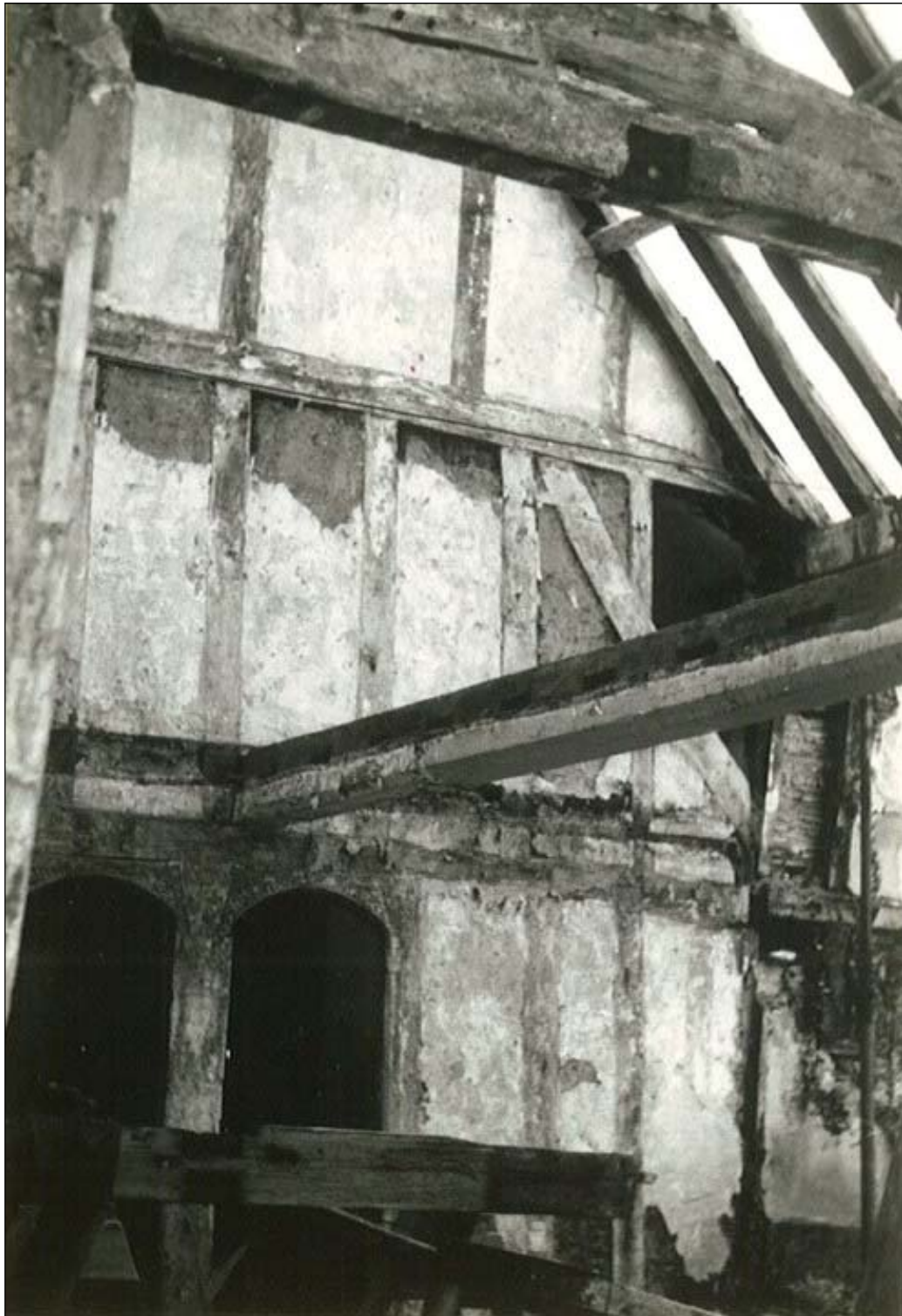
The interior of the hall during restoration looking towards the low end, with an iron girder that latterly supported the first floor still in situ. Panels of 15 th -century wattle and daub were retained in this wall.
