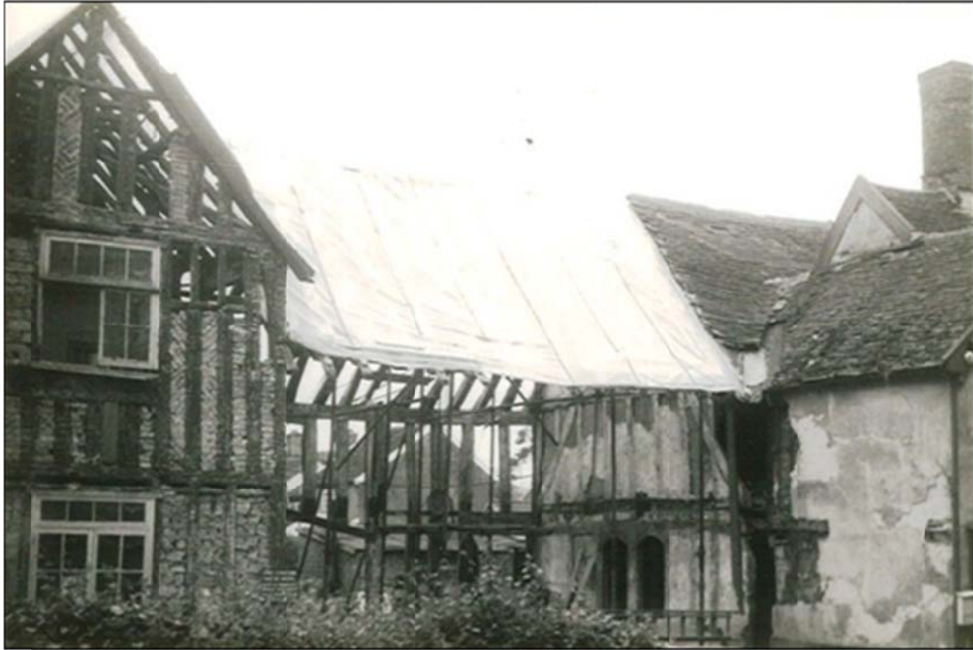
The hall stripped back to its frame. The service doors to the low end can be seen in the right hand wall. Note the neat brick infill to the first floor panels.
