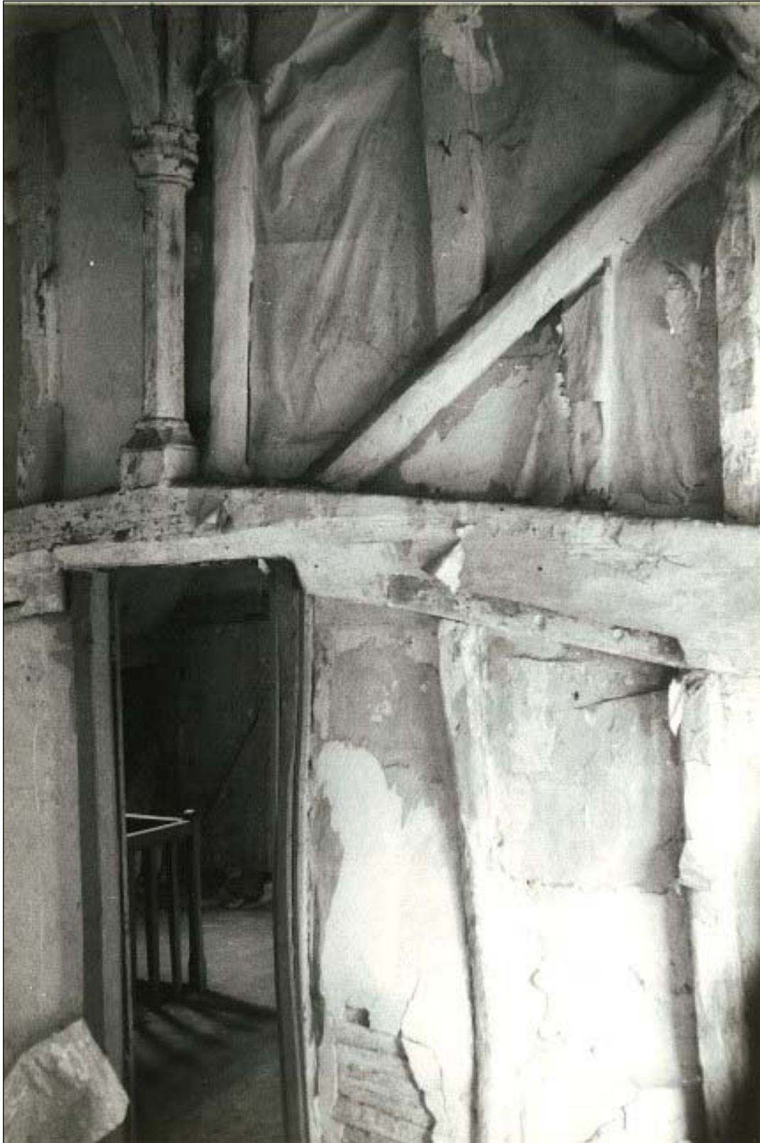
Crown post and tie beam of the hall before repairs. The tie beam beneath the crown post has been cut to give head room and the crude work of the inserted partition on the line of the open truss can be seen very clearly to the right of the crown post.
