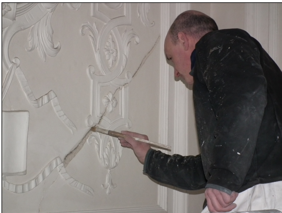
By 2013, cracks had opened up in The Music Room, requiring specialist repair skills.
