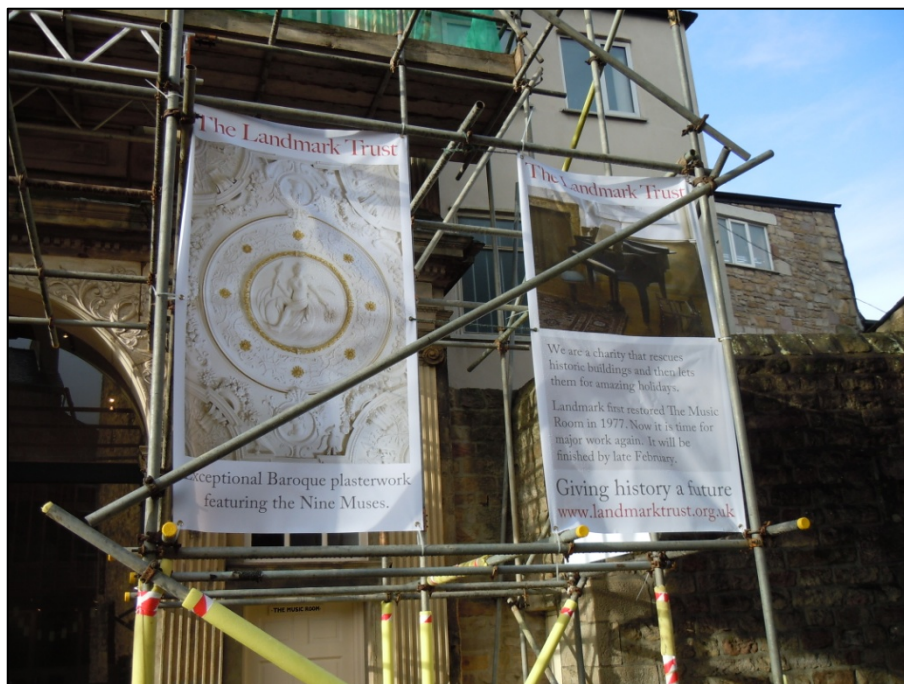
Scaffolded for the 2013 works, the Music Room doubled as an outdoor gallery.
