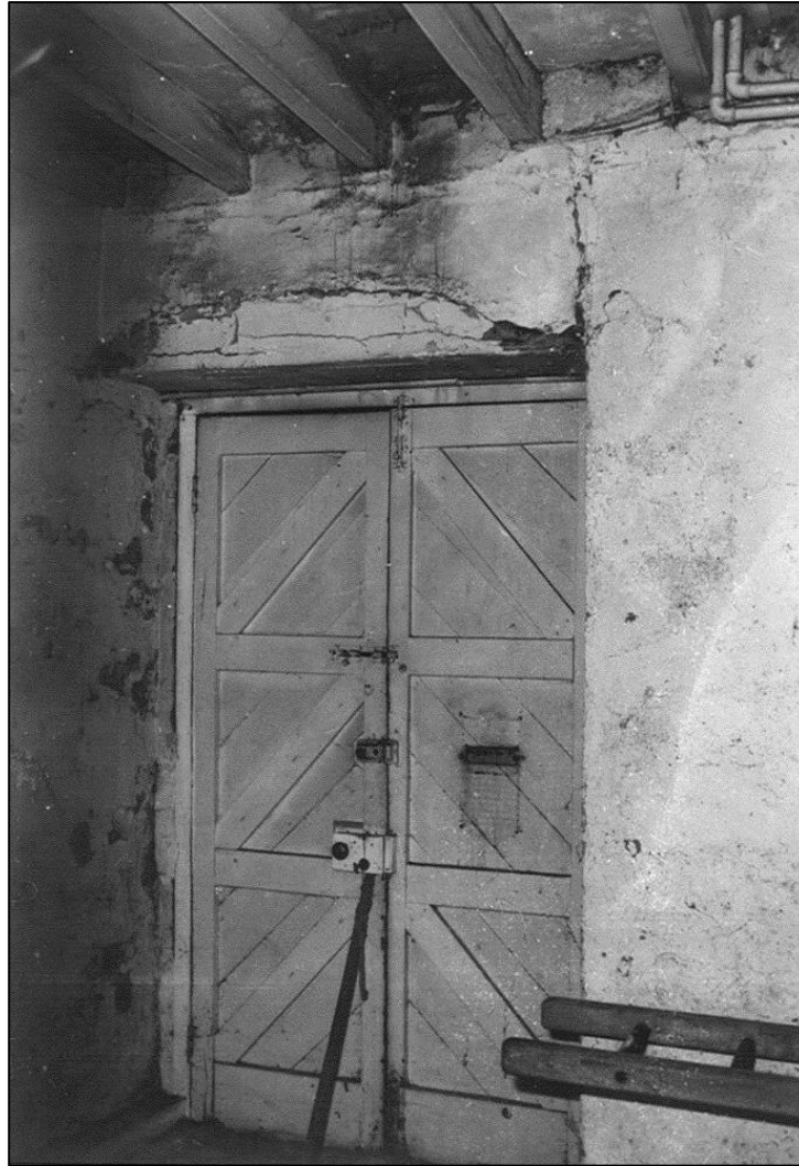
The former front door in the south east wing. You can see damp penetrating the walls causing damage to the plaster
