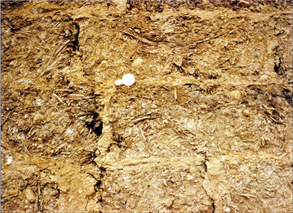
A detail of the clay daub on the east end of the farmhouse.
