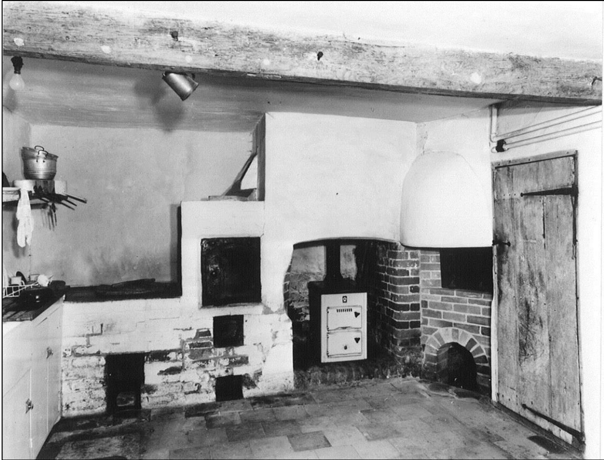
The kitchen as it was in 1979. A lot of damp was coming through the chimney wall.
