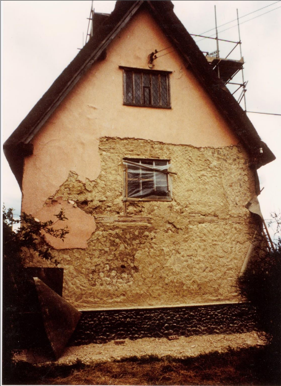
A bulge in the wall at the east end had caused the plaster to crack more than elsewhere so that it no longer formed a secure base for the coating of limewash.
