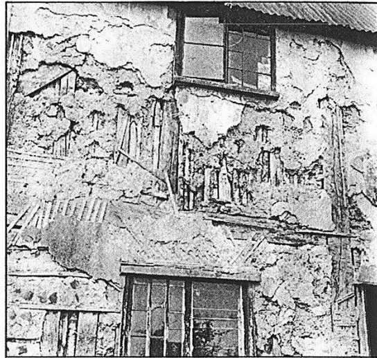
Exterior wall before repair.
