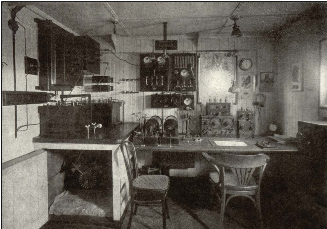
An early, 1.5 kilowatt Marconi transmitter. Similar equipment may have been installed in the top floor of the Tower.
