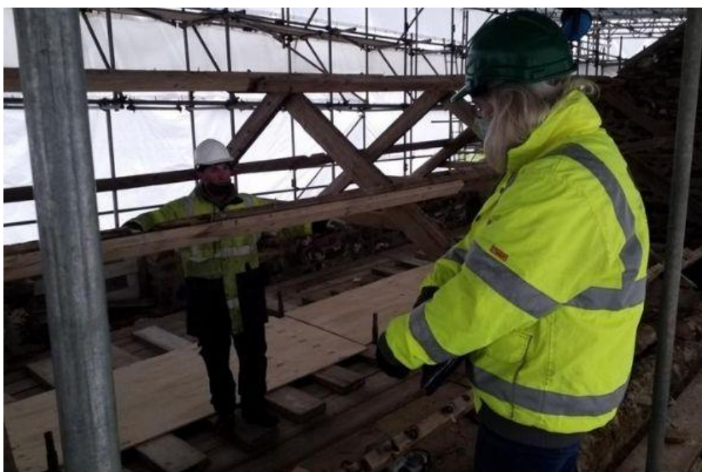
Contractor Paul Carter and structural engineer Kathy Gee in conversation under the scaffolding that enclosed the roof structures.
