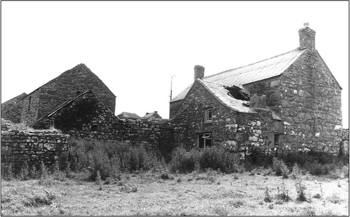
The dairy (or bakehouse?) needed some rebuilding. The ground floor window had been enlarged, with a modern frame; but has now been made smaller again
