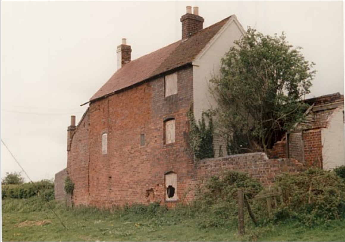
The different coloured bricks which show the various stages of alteration and addition are clearly seen here, on the now inaccessible back walls of the cottage, photographed before repair.
