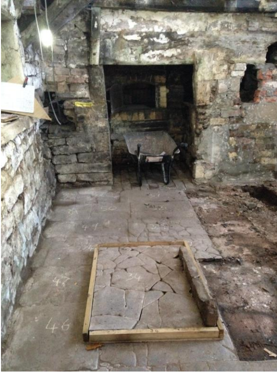
The ground floor was carefully lifted piece by piece ready for the installation of underfloor heating (here in the rear kitchen)
