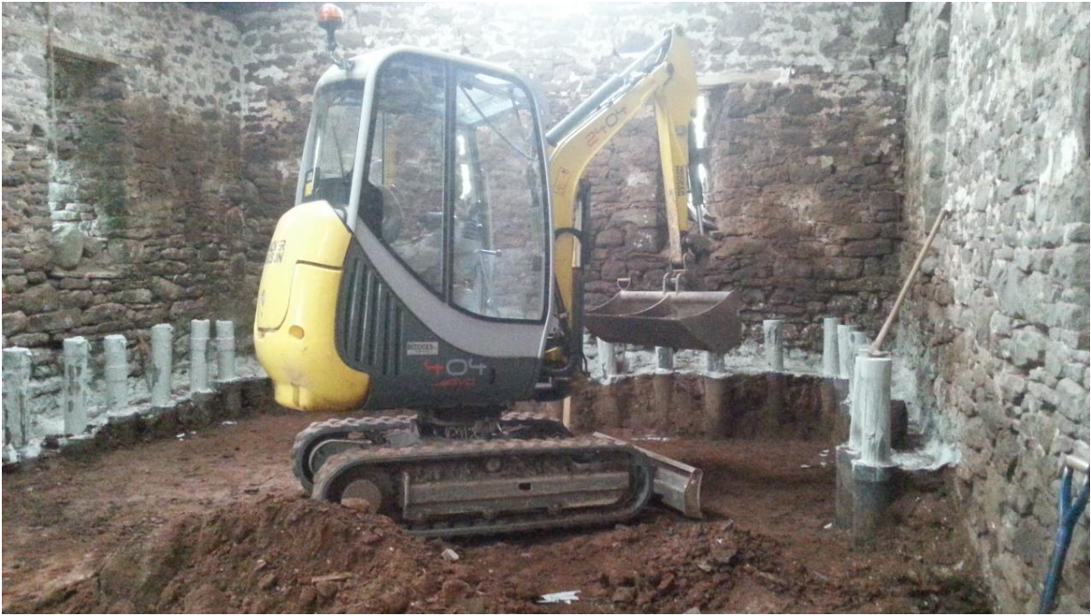
Major piling and underpinning underway in the Threshing Barn, today invisible beneath the concrete plinth that also helps stabilise its walls. The excavation of the floor also enabled the installation of underfloor heating.
