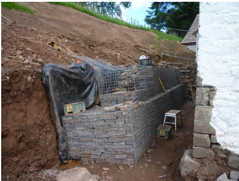
Huge gabions have been installed against the west bank behind the solar range, serving both to improve site drainage and to act as a retaining wall.
