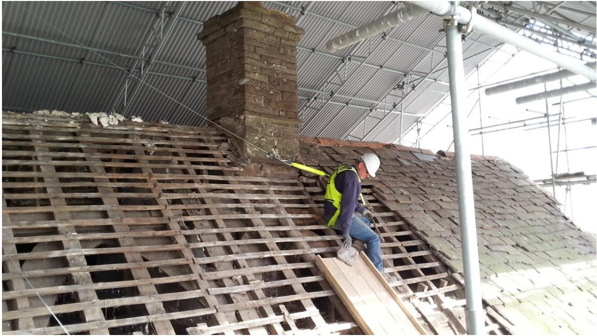
Autumn 2016. When the roof was stripped, each tile was individually removed by hand, and passed down a chute just as it would have been in centuries past.
