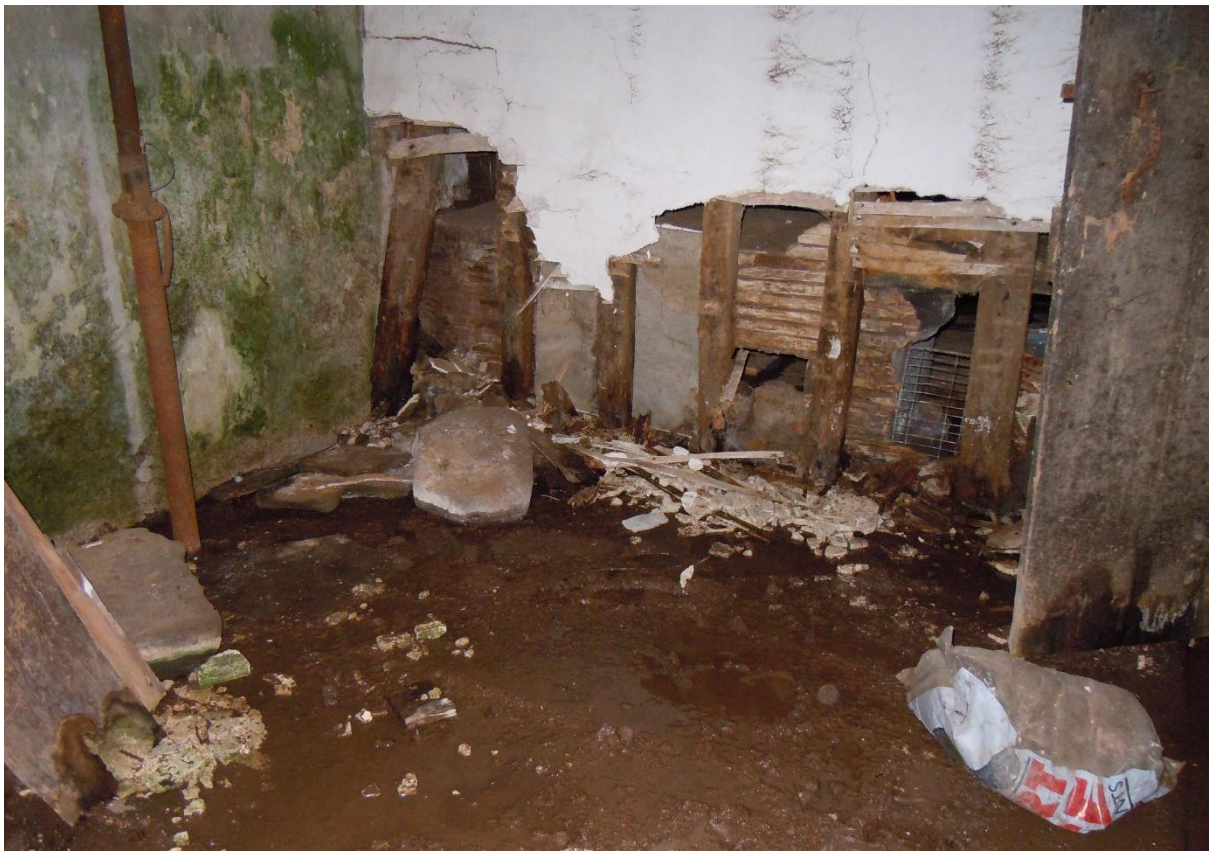
There was standing water in today's solar end bedroom (top). Today's ensuite bathroom was equally un-usable (above).
