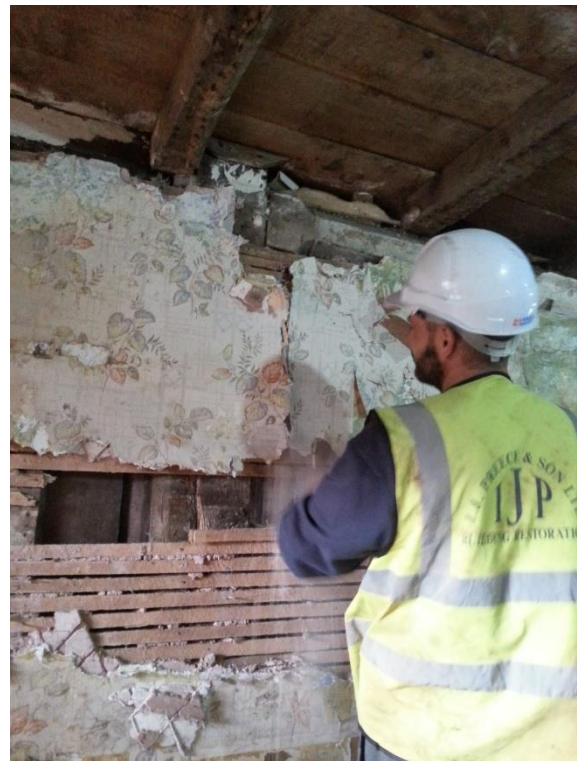
John Goom (architect) and Tom Hill (structural engineer) scrutinise the roof of the solar range, whose timber was felled in 1418/19. Meanwhile, we were opening up to investigate the spere truss in the cross passage.
