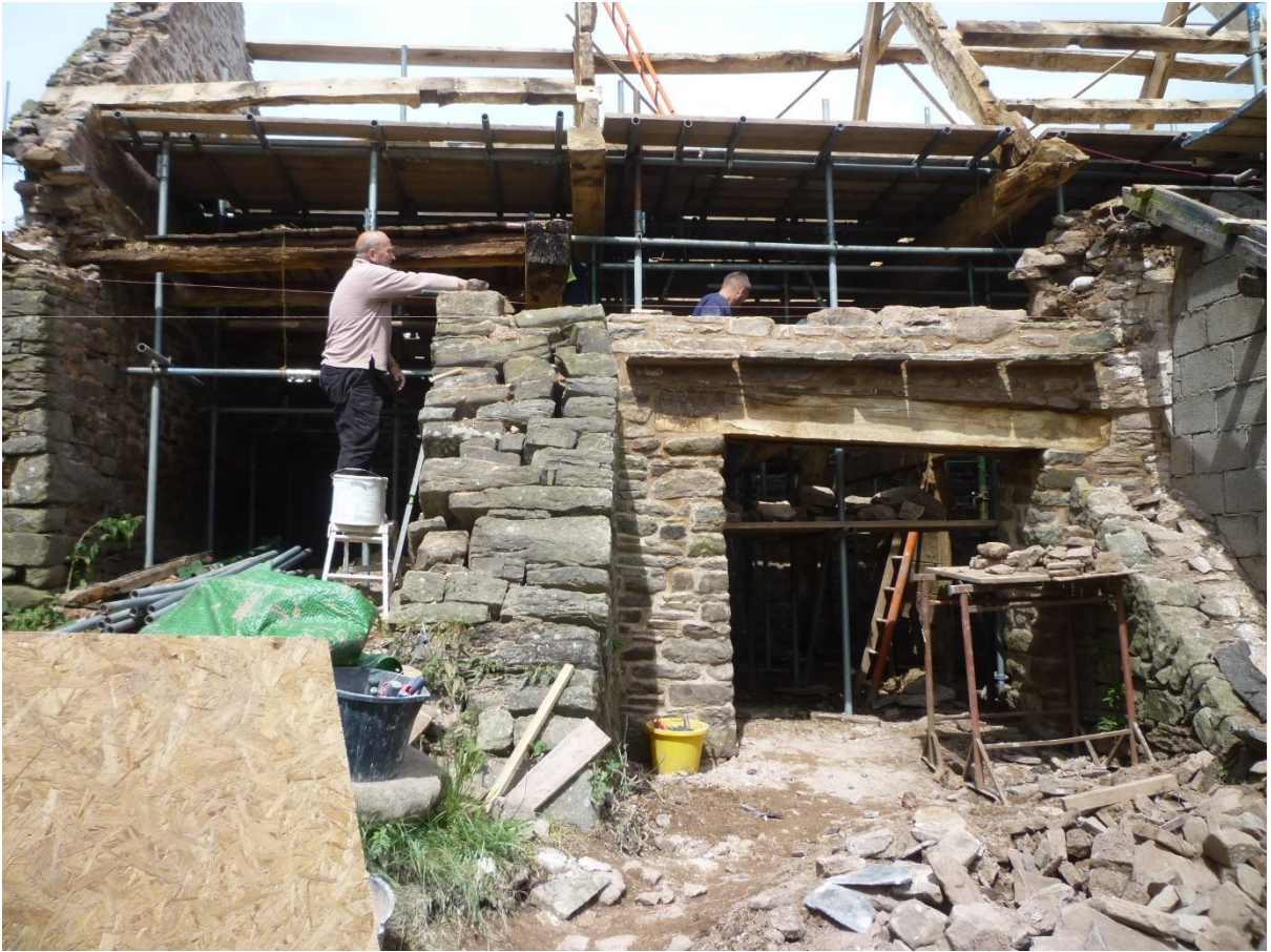
Attention also turned to the outbuildings. Here, the Beast House roof is stripped ready for re-battening. Its north wall has been rebuilt by now. We learnt that the little lean-to shelter is much older than we had thought.
