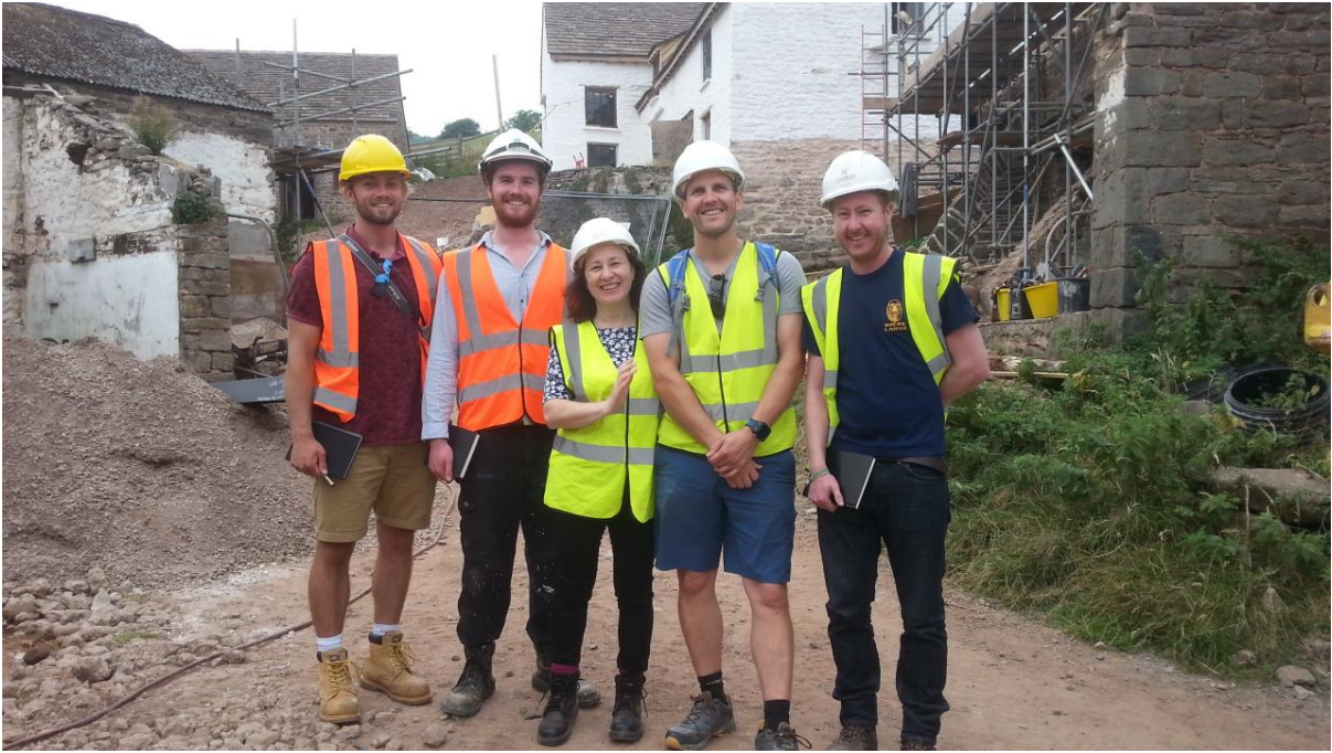
The 2017 SPAB Fellows visited the site in September, here with Susan McDonough, Landmark’s Head of Historic Estate. By now, the underfloor heating had been installed and limecrete floors were down in the house (below in the hall).
