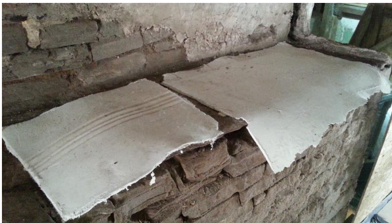
Trial samples of moulding ready for approval, and the plasterer's tools. The wooden mould will be dragged through the wet plaster to form the moulding.
