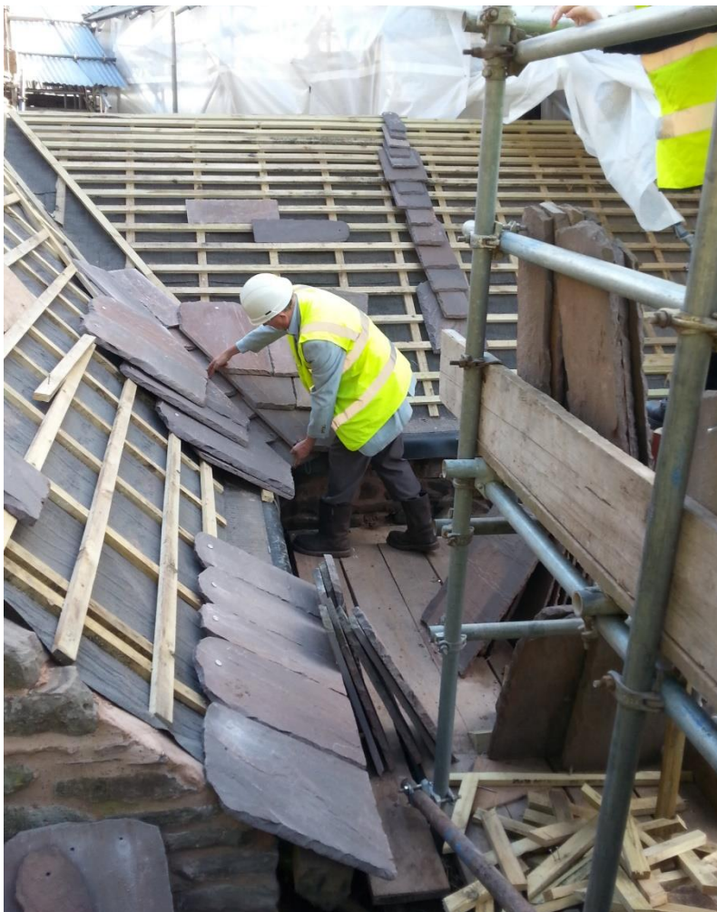
Project architect John Goom laying out a Welsh valley, a traditional solution to making the junction between roof slopes watertight. The massive stone tiles, which run in diminishing courses from the roofline, are Devonian Old Red Sandstone. They were quarried from near Longtown. Where sound, salvaged tiles were re-used among the new ones.
