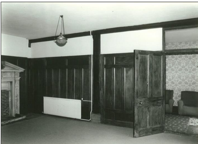
Right: The plaster decoration of the ceiling surround, although damaged by partition walls. It seems that there never was a cornice.
