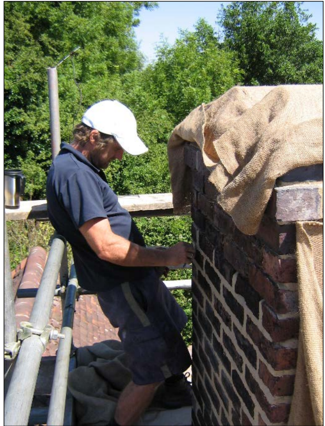
Pointing the chimney stack. At the height of summer, as here, lime mortar must be protected by damp hessian to prevent it drying out too quickly and cracking.
