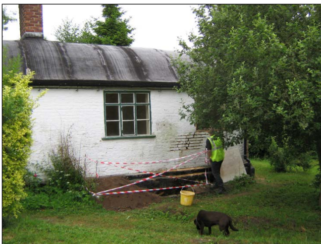
Position of one of the stitched cracks.
