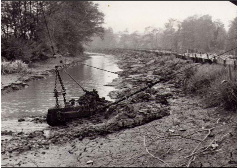
Dredging at Lapworth in April 1961. Note the mud boards along the towpath. (SCS)
