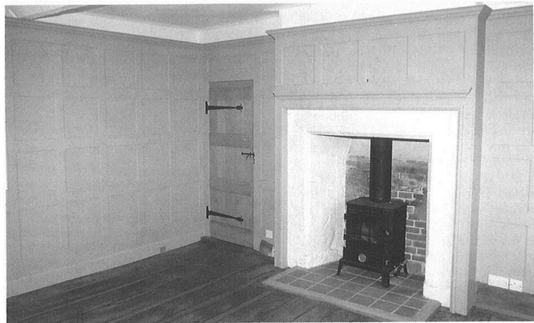
In the room over the gateway floorboards were repaired using the methods described in SPAB Information Sheet 10 "Patching Old Floorboards" by Philip Hughes.
