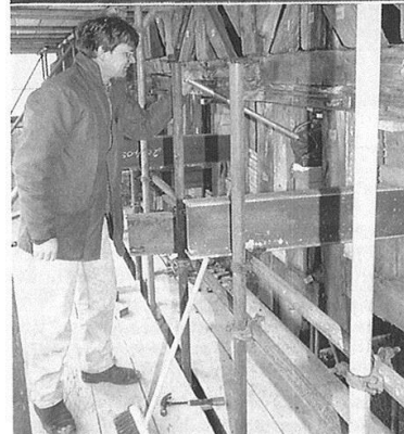
Hydraulic jacks were used to remove eight of the 12 inches of subsidence in the east wall.
