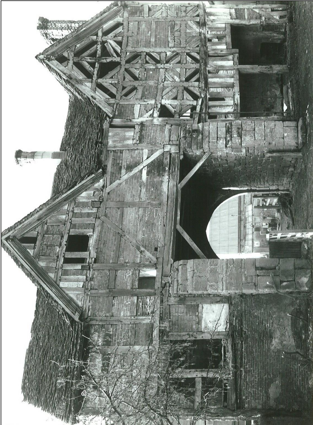
The east front before repair
