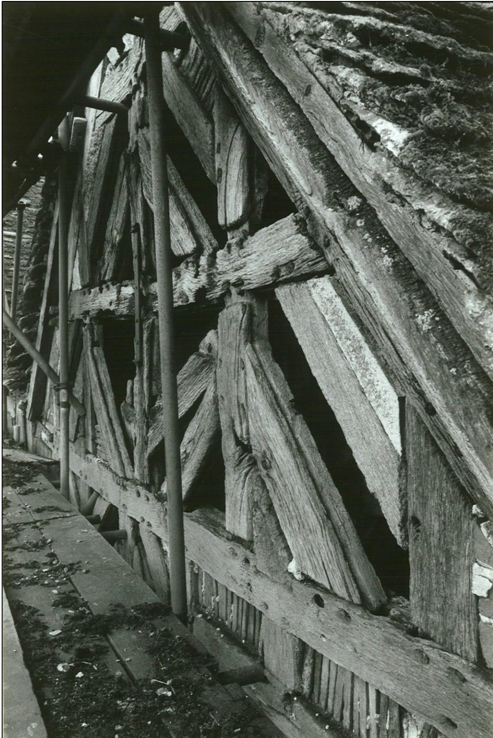
The condition of the north east gable
