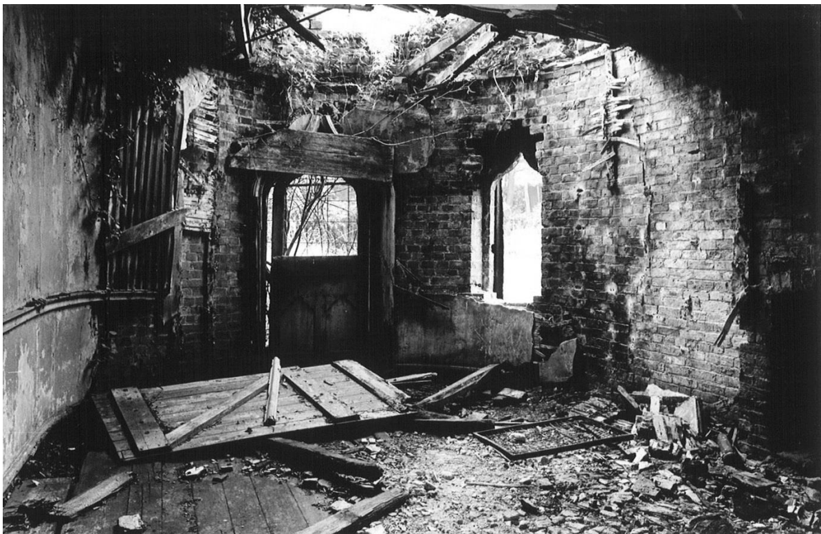
The garden room showing further decay in 1988.
