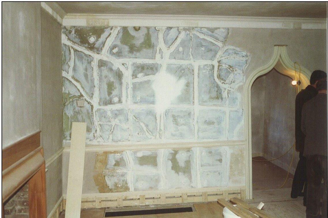
Old plaster refixed to the walls, and integrated with the new; also old, darker, pieces of cornice.
