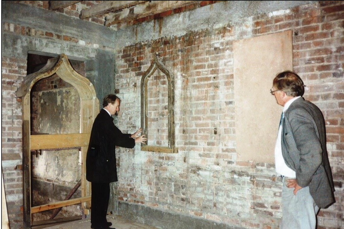
Mike Kent of Rodney Melville & Partners (left) checks the position chosen for the new window.
