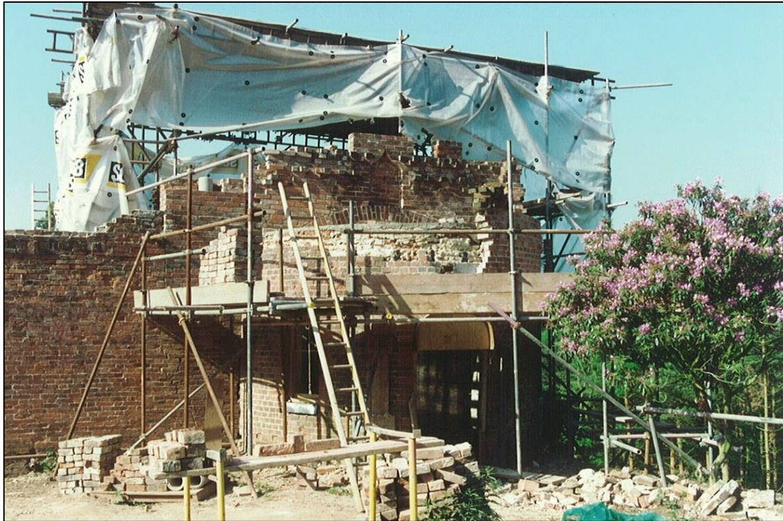
The summer house ready for repair. Secondhand bricks were used for rebuilding the parapet alongside those salvaged from the site.
