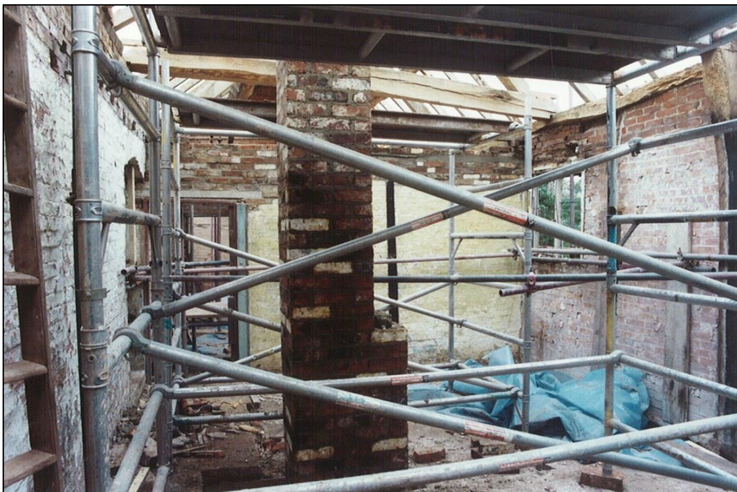
Looking from the single bedroom to the present bathroom. Both ceilings and partitions in this part of the cottage were too decayed to repair and had to be completely renewed.
