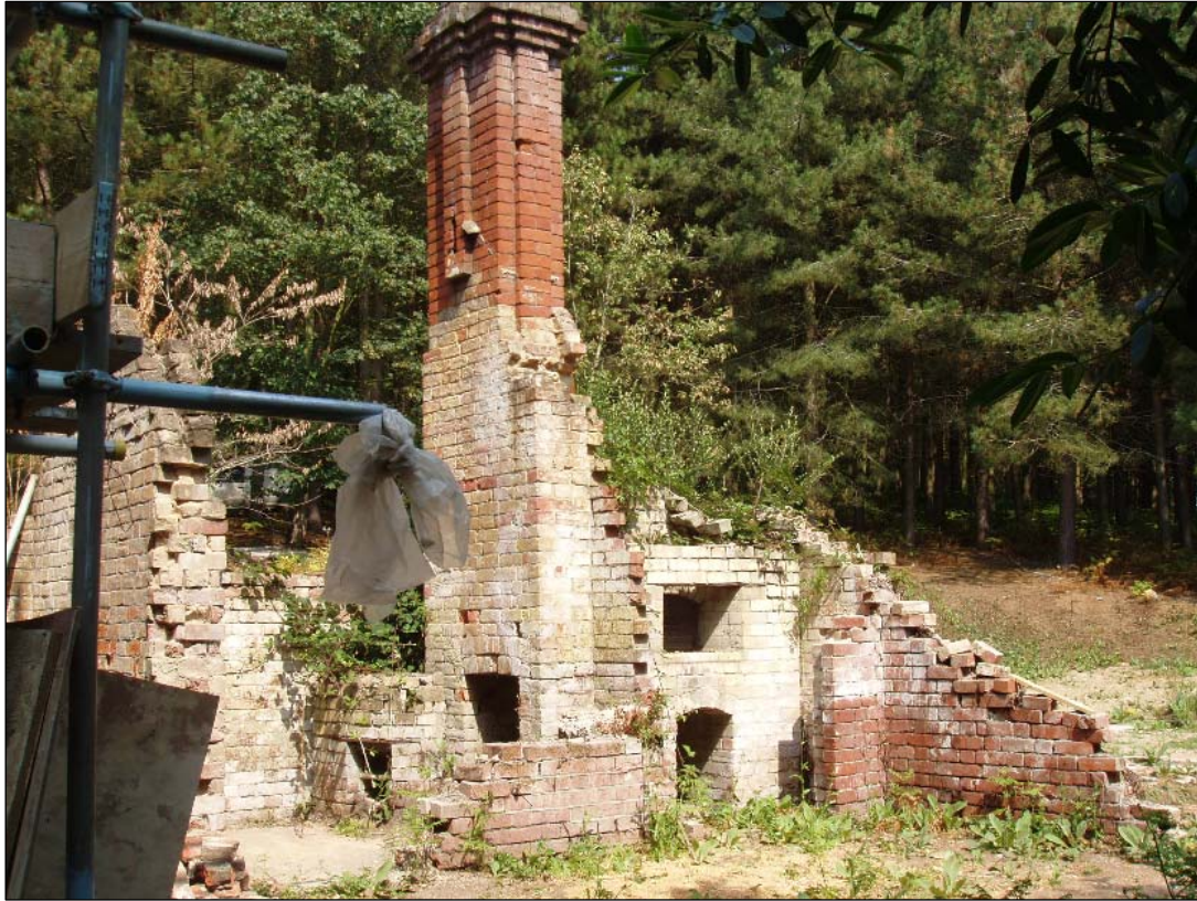
The washhouse before work began. A bread oven had been inserted at a later date into the space occupied by the earth closet shown on Usher's plans.
