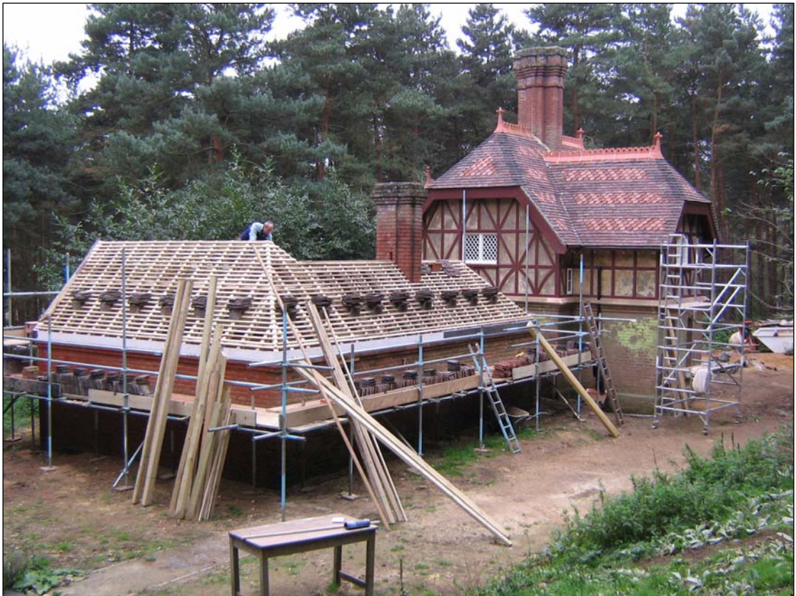
The repair of the exterior of the cottage complete, we decided to reinstate the outbuildings, using John Usher's original designs.
