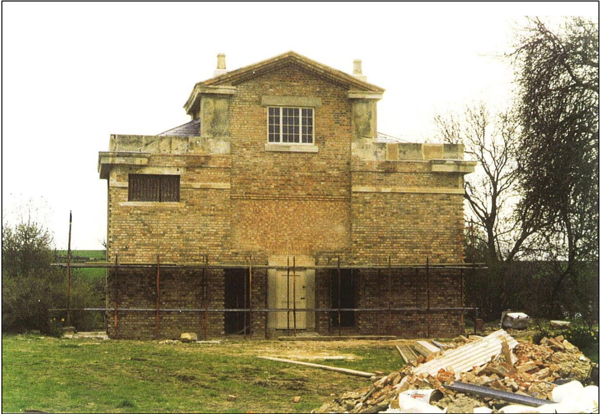
The House of Correction during repair and conversion, the 1930s extensions now removed
