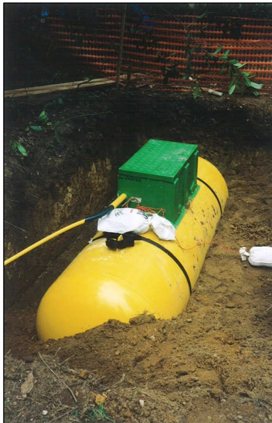
The buried gas tank
