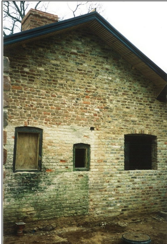
The courtyard wall with the bedroom extension removed and the window inserted
