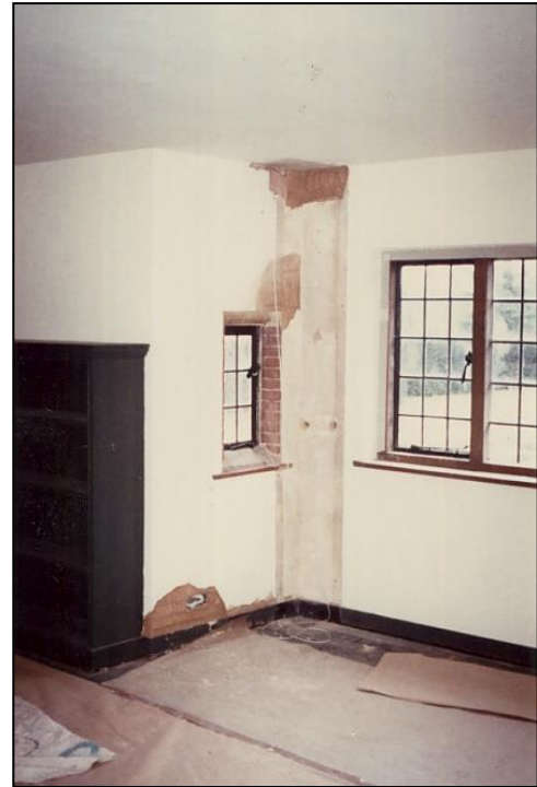
In the library the pipes from the granny flat were removed. The larger window in this picture is the addition of c.1930.
