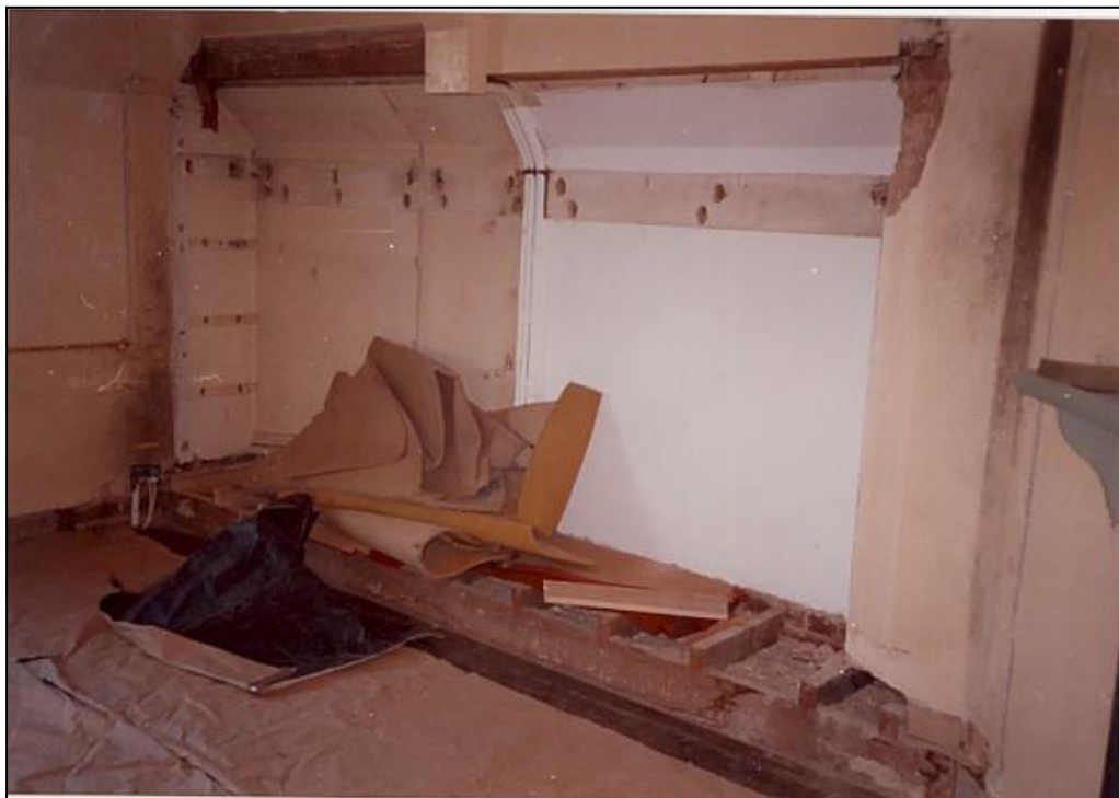
Bedroom no. 7 showing the raised bulkhead over the kitchen window after removal of the fitted furniture.
