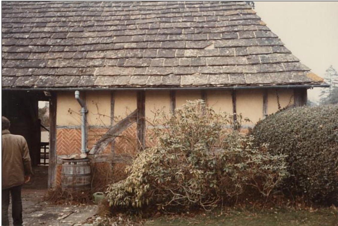
The North Barn. The south wall had rotted behind the water butt.
