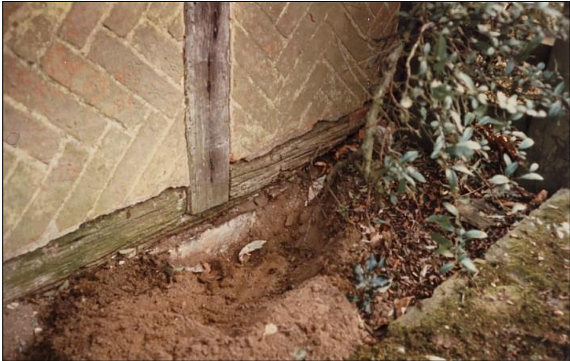
The sole plate and brick panels in the north west corner were replaced.
