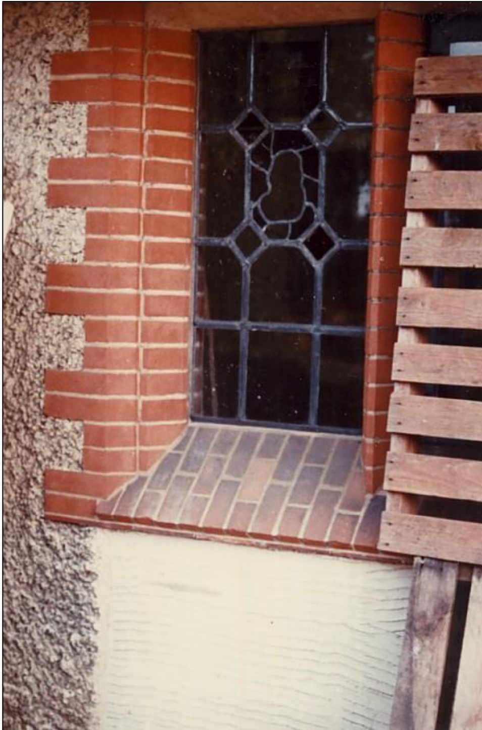
The render on the north wall below the parlour window needed repair. Here the scratch coat has been applied.
