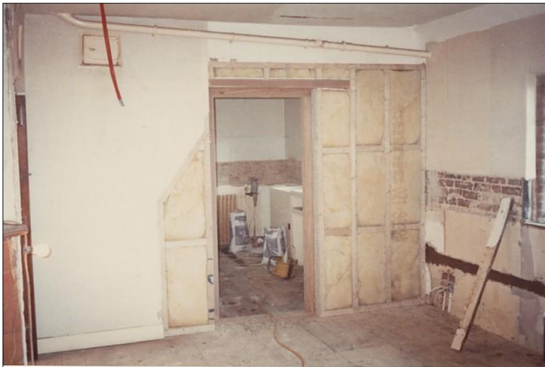
The parlour with the partition back in its original position and the fitted cupboards and sinks removed.
