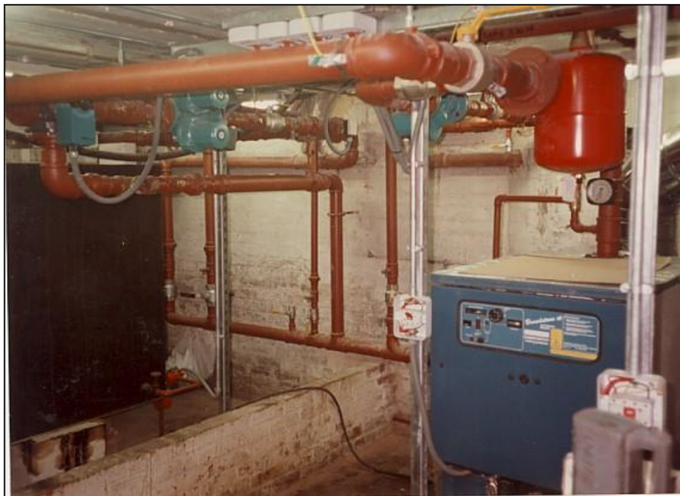
The new boiler.
