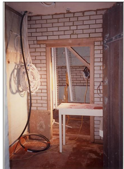
The new partition seen from the back door. The cable drops are for lighting and security.
