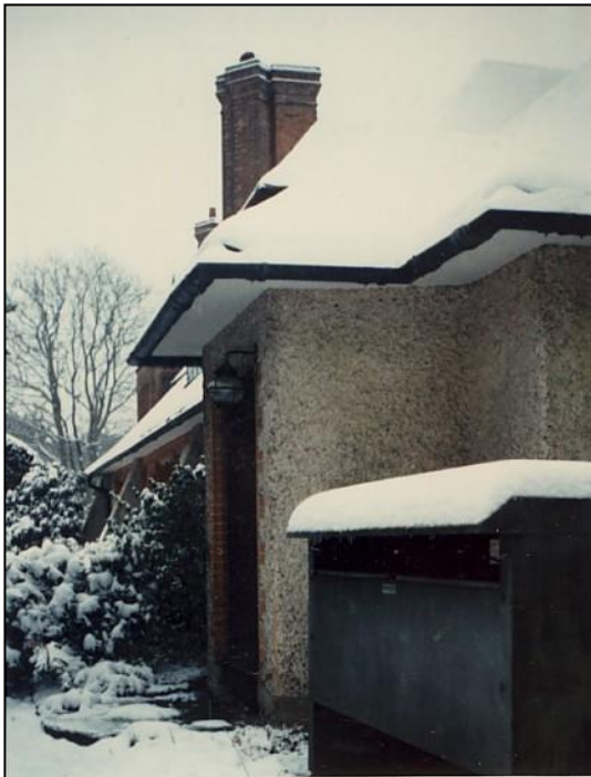
Boarding below the eaves had to be replaced. The heat exchanger in the foreground was part of the old central heating system and has now been replaced.
