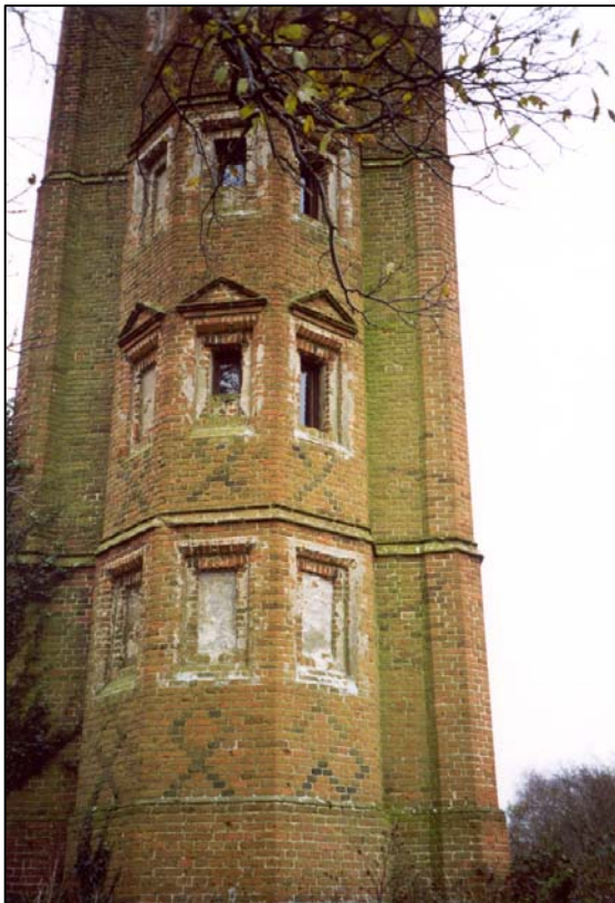
The sad state of the exterior
